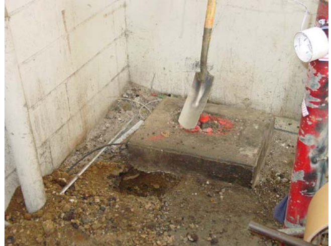
PHOTO 2. Concrete dispenser foundation located west of the block building. The sample identified as "Dispenser" was collected adjacent to the foundation.
