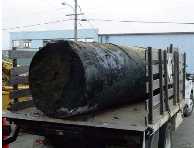
PHOTO 5. Tank is secured onto truck bed prior to its transport to Ecology Control Industries in Richmond, California.
