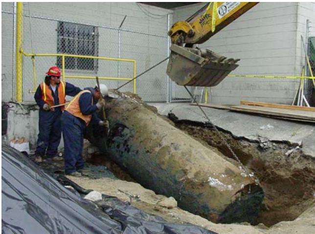
PHOTO 3. Tank is shown as it is being lifted out of pit by excavator.
