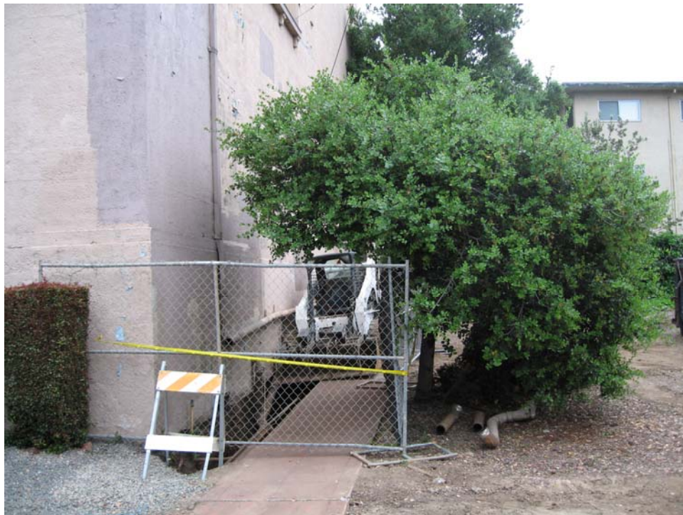
Parsons – Piedmont: Photo 04 – Removal Complete, 408 Linda Avenue, Piedmont, CA. Photographed by: T. R. Winsor
