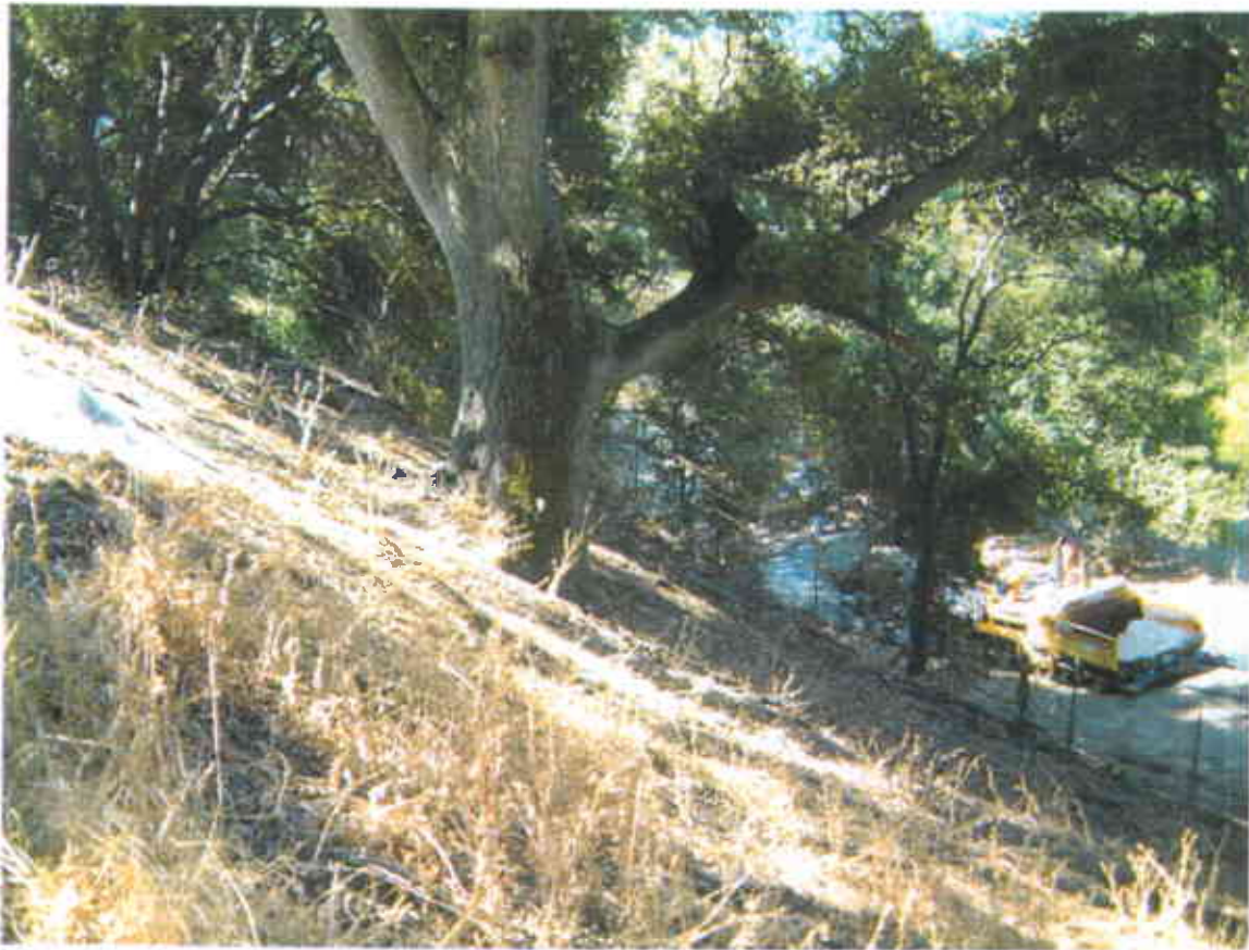
Figure 1. The steep 84 percent slope immediately below the pipeline break (looking south and down slope towards Calaveras Road)
