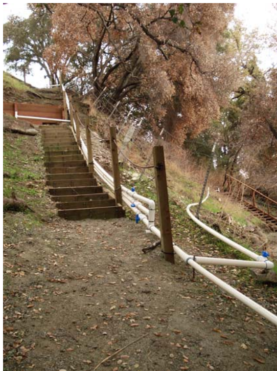
Photo 8 Piping Manifold, SVE-6 through SVE-9
