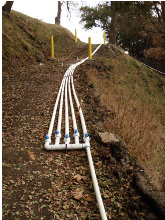
Photo 7 Piping Manifold, SVE-1D through SVE-5
