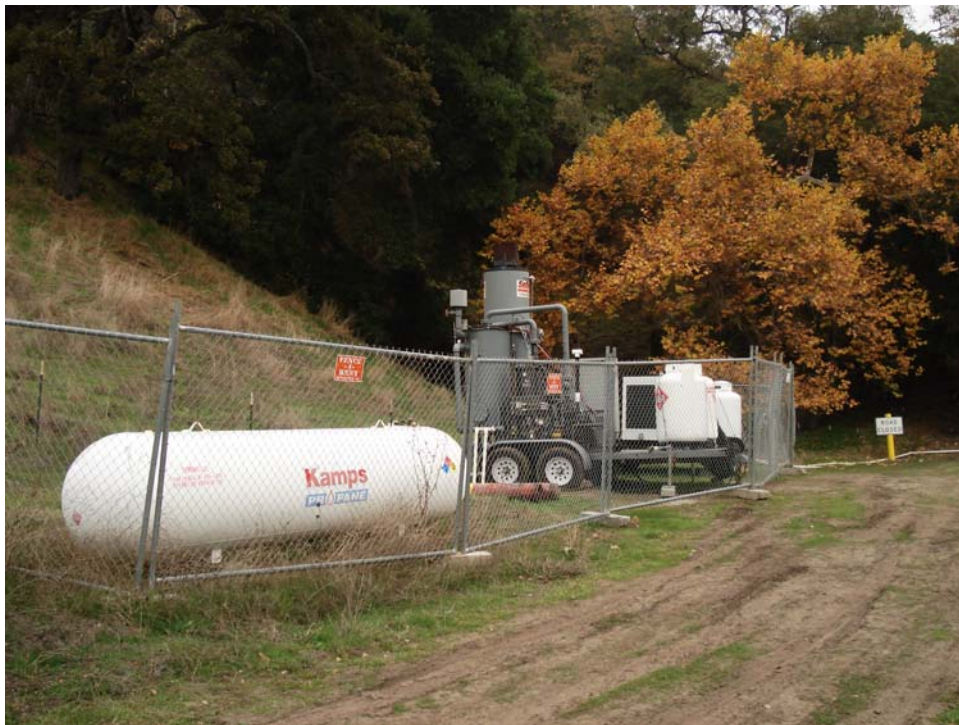
Photo 6 SVE Treatment System
