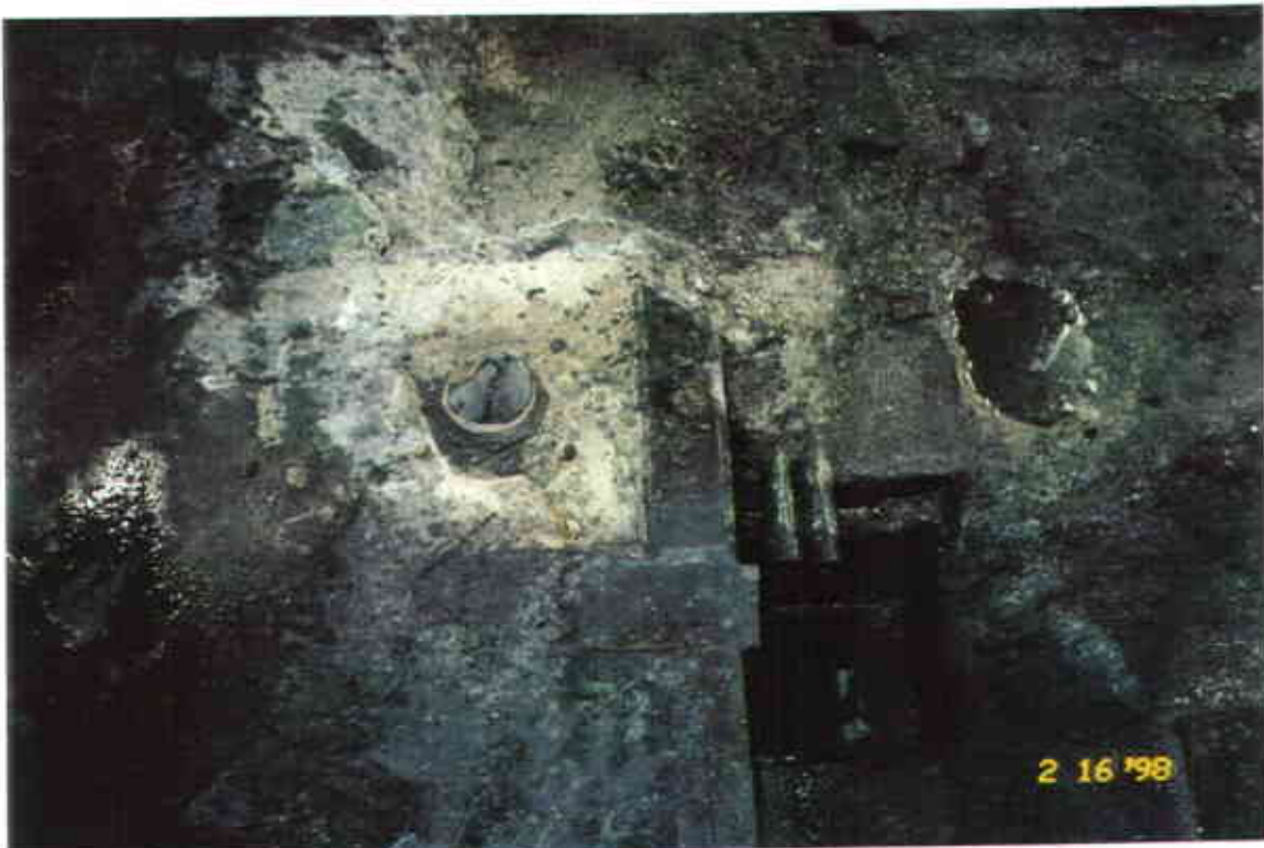
Photograph 6 - Milling Machine Pit Exit Pipes
