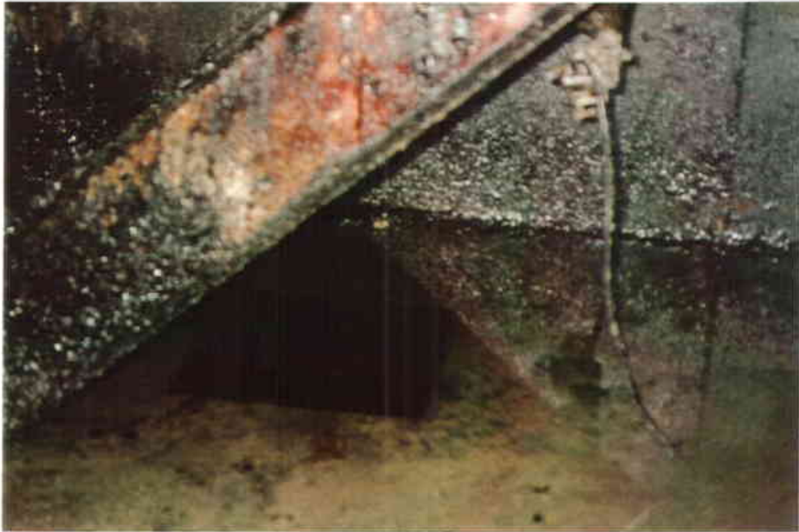
Photograph 3 - RAFFEX Tank Vault Sump
