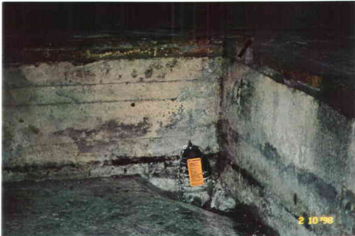
Photograph 4 - Camelback Conveyor Pit Plug inserted in exit pipe; arrow pointing to crack in floor.
