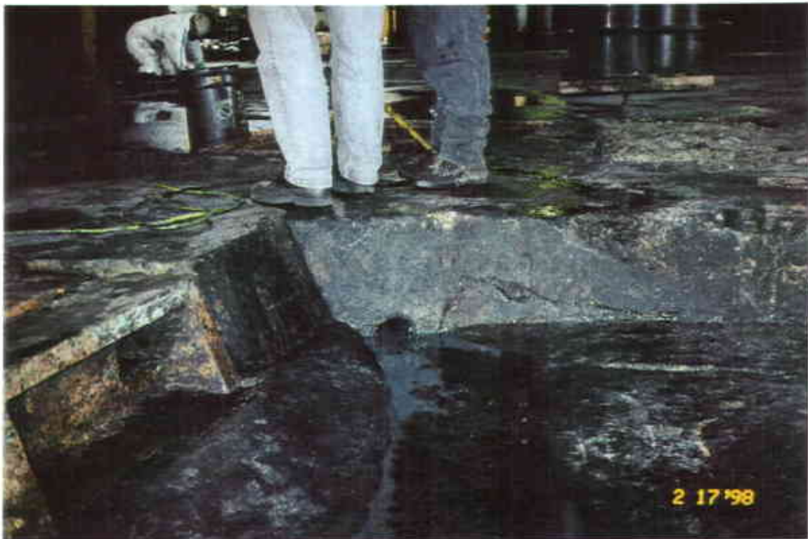
Photograph 5 - Milling Machine Pit Exit Pipes
