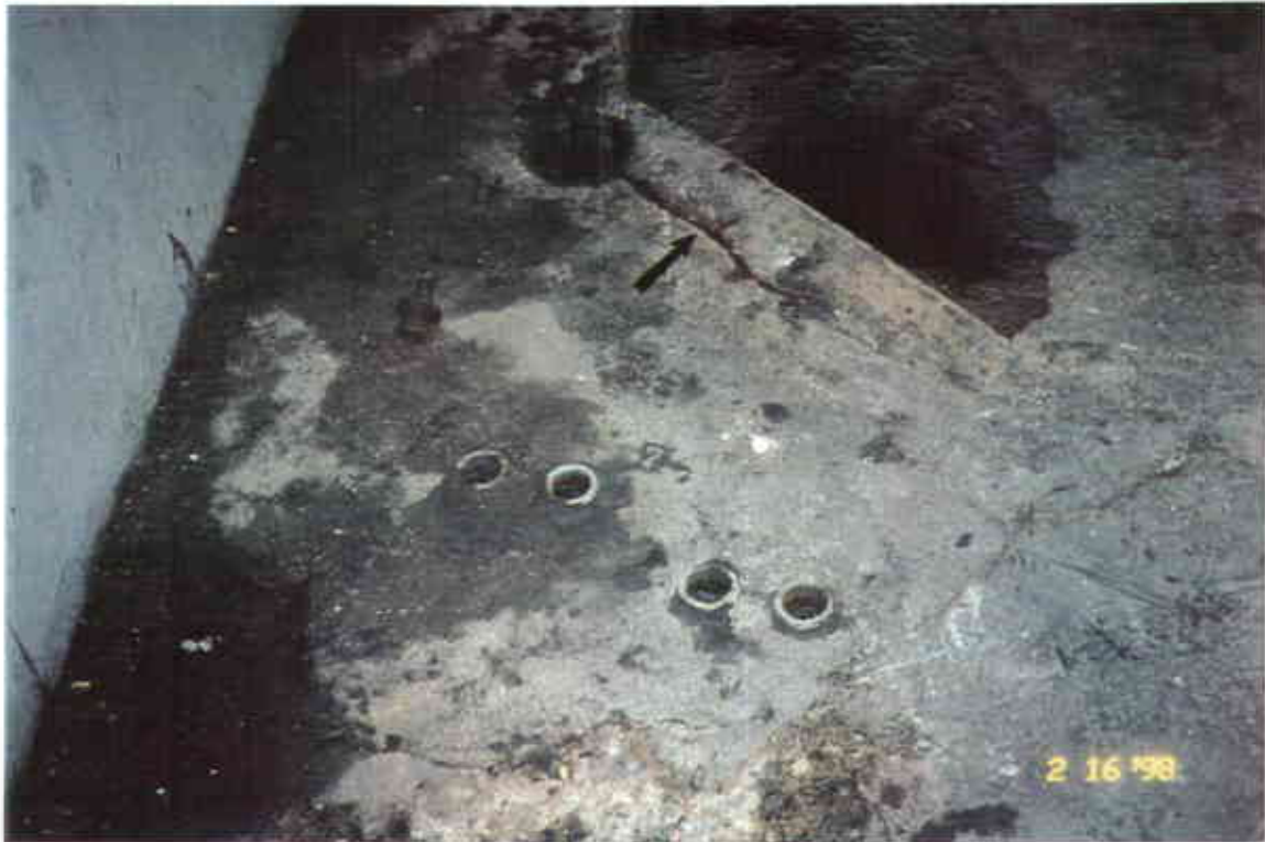
Photograph 7 - Milling Machine Pit Crack
