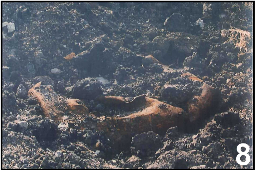
Close-Up of Top of UST April 15, 2004
