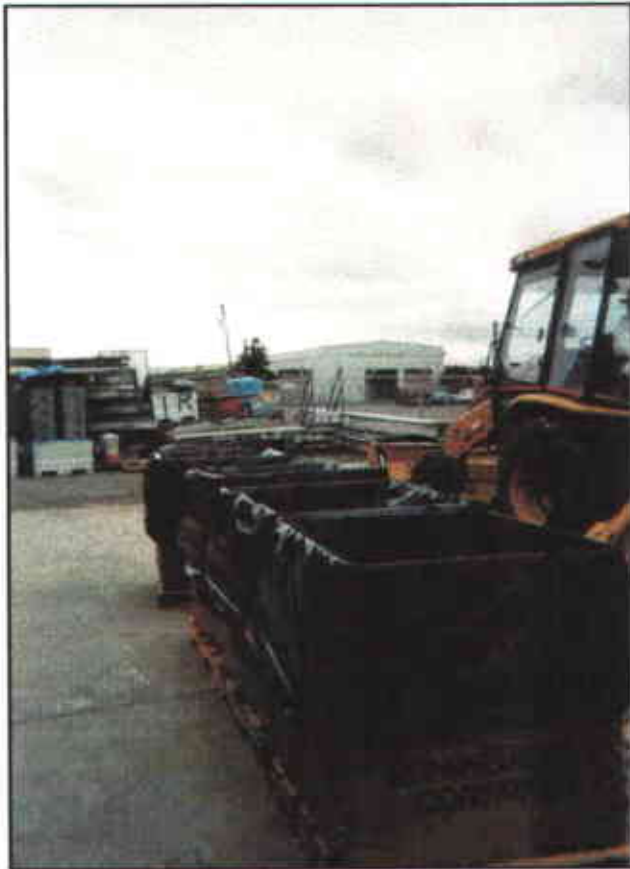
Photo 2: View looking east of tri-wall containers used for disposal of excavated soil.
