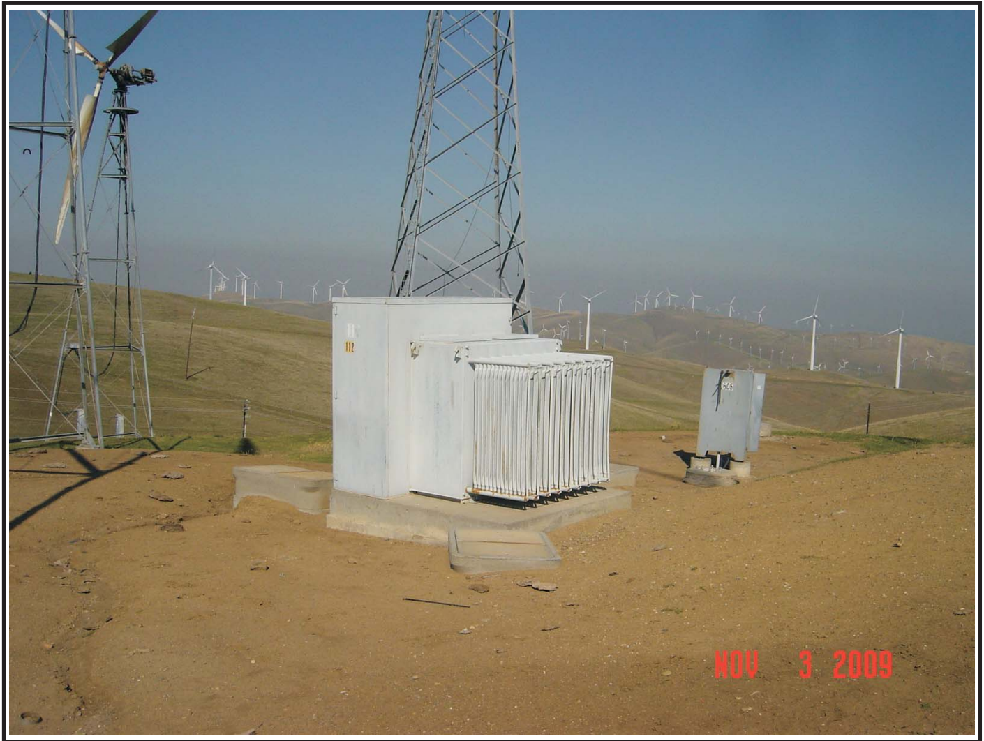
Transformer 112, view looking west. Note the radiator which contains the transformer insulating oil on the right hand side.
