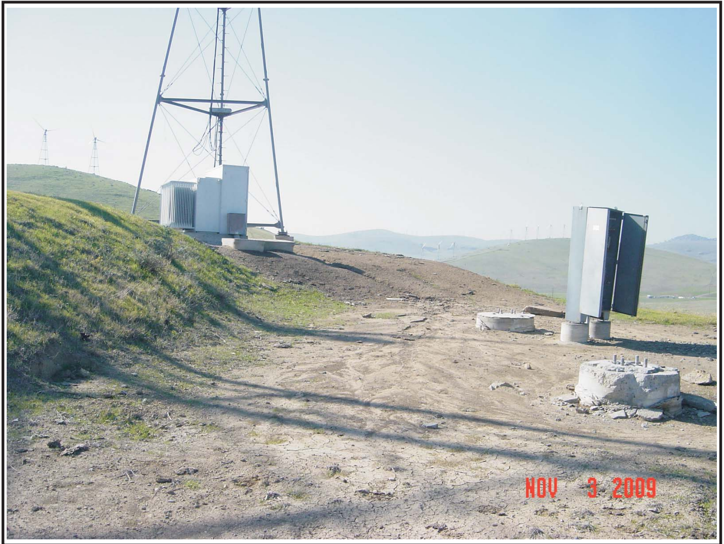
Transformer 112, view looking west. Note the grade change which resulted in the oil flowing east and pooling in the flat area below.
