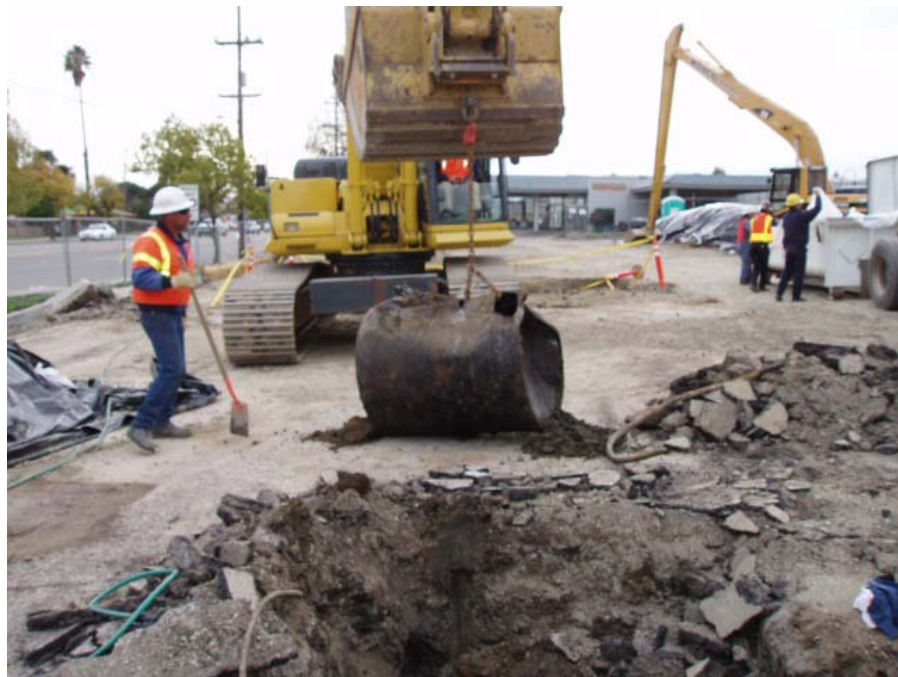
Photograph #2: Tank as it is being removed from the ground. The hole located at the top right corner was caused during excavation activities, prior to knowledge of the tank.
