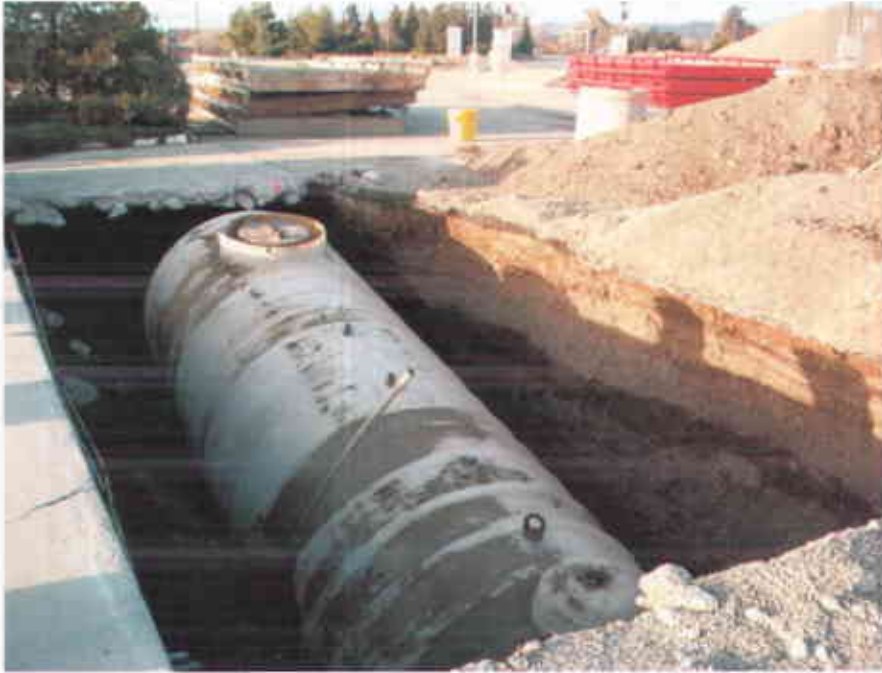
Gasoline Tank Exposed
