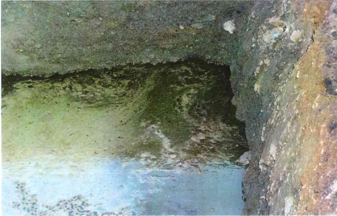
13. Floating product on the surface of water in the excavation for UST No. 8
