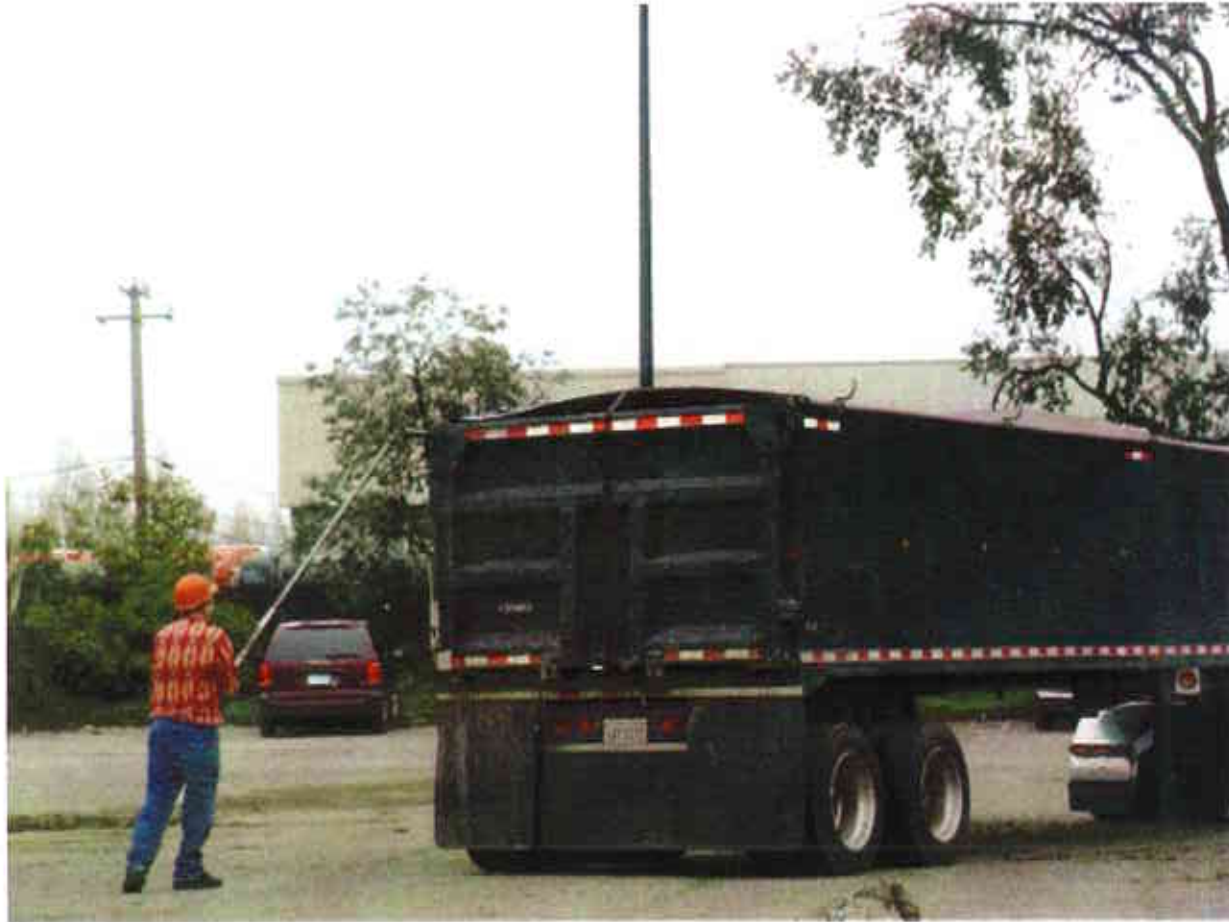
33. Covering the trucks loaded with soil prior to trucks leaving the site
