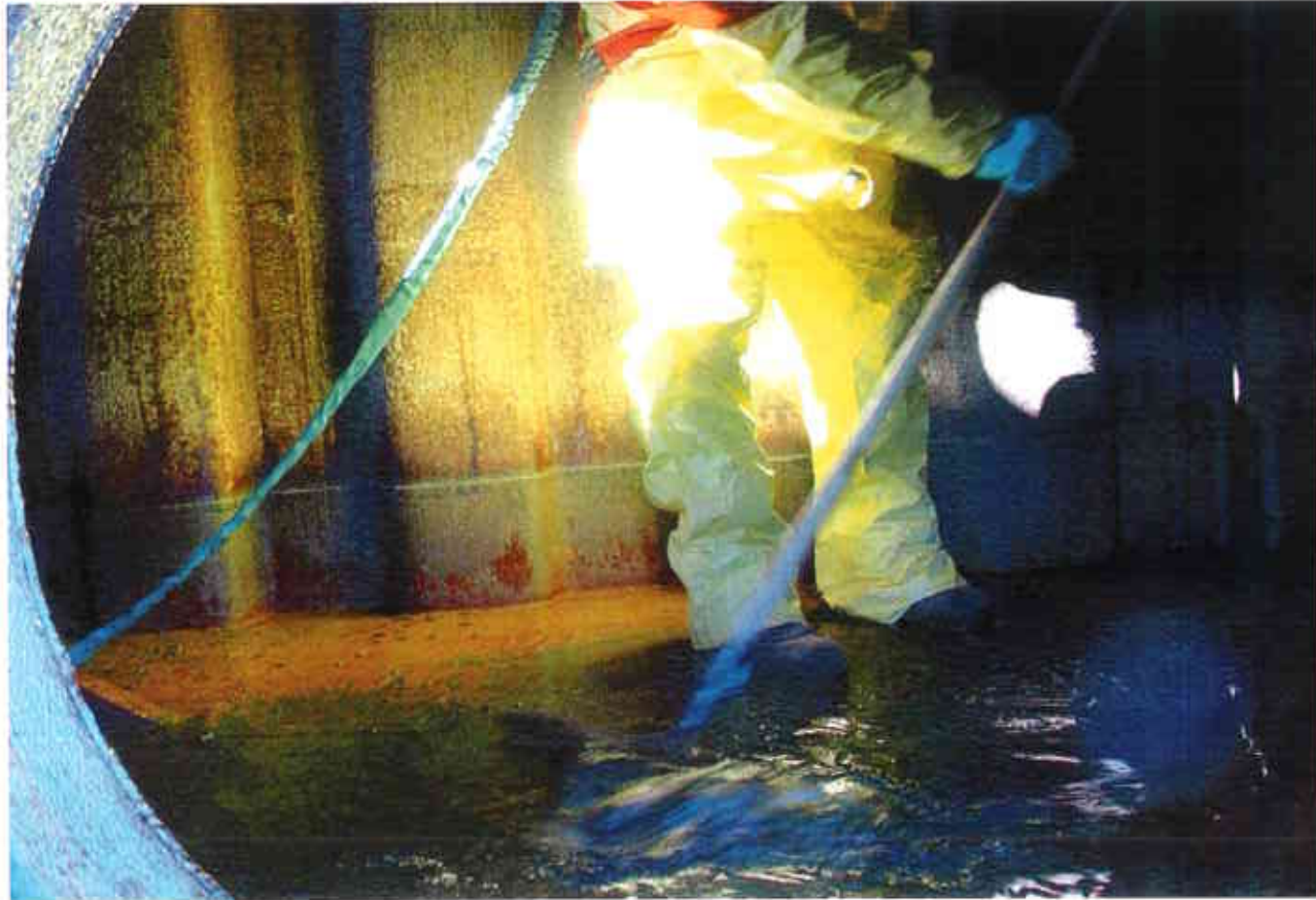
31. Manual rinsing and cleaning of the interior of the tank prior to its removal from site
