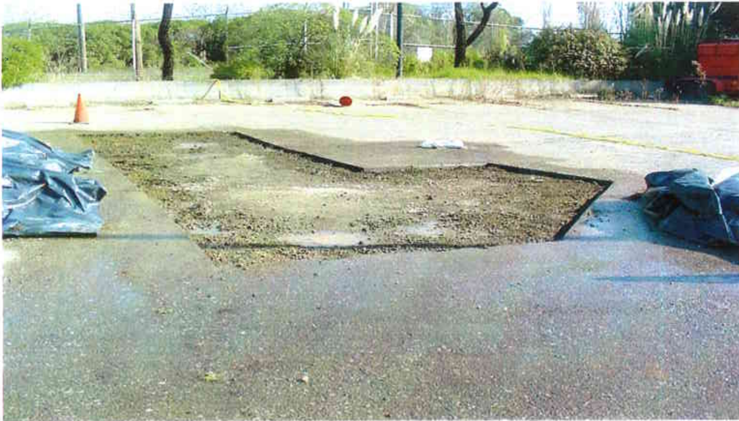
24. Smooth pavement edges produced in the UST No. 8 location prior to paving
