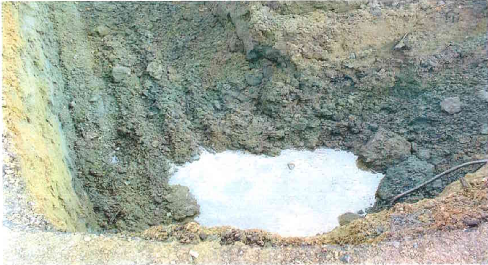
9. Water accumulation in the excavation
