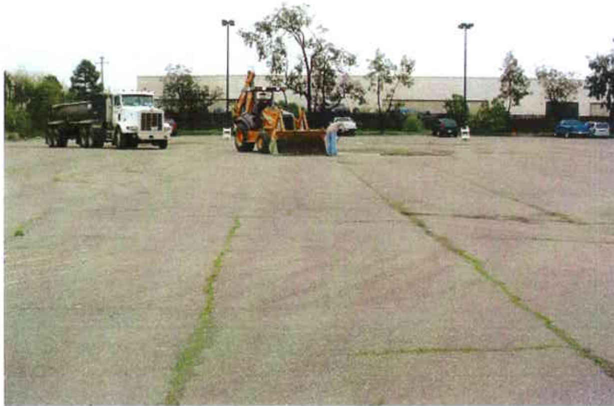
37. A view of the site after removal of the water storage tank and stockpiles of excavated soil and asphalt debris, but prior to repaving
