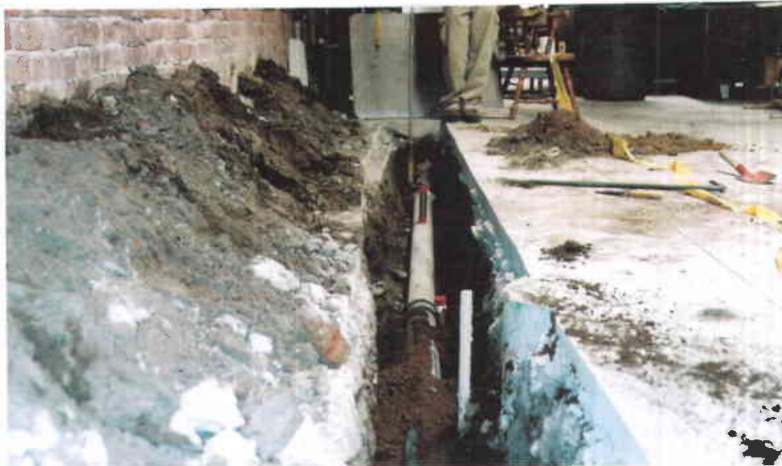
Subject: Sanitary sewer line trench, looking to the north, showing hand auger sampling locations (steel tubes with red caps)
