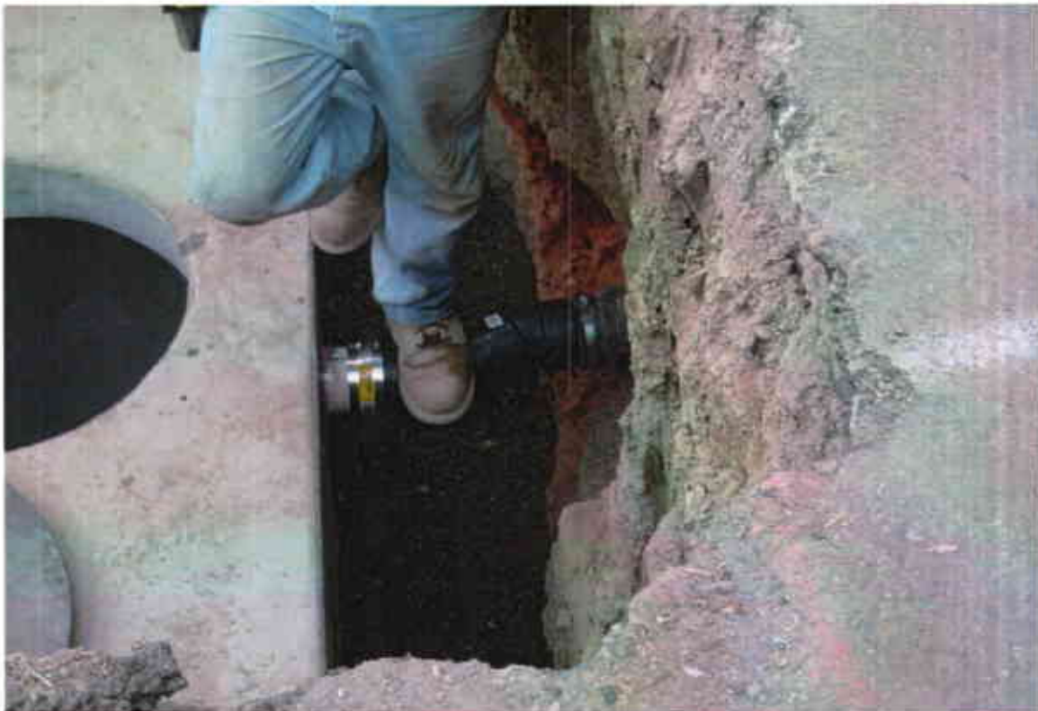
Photo #10: View of the existing piping being reconnected to the new OWS.
