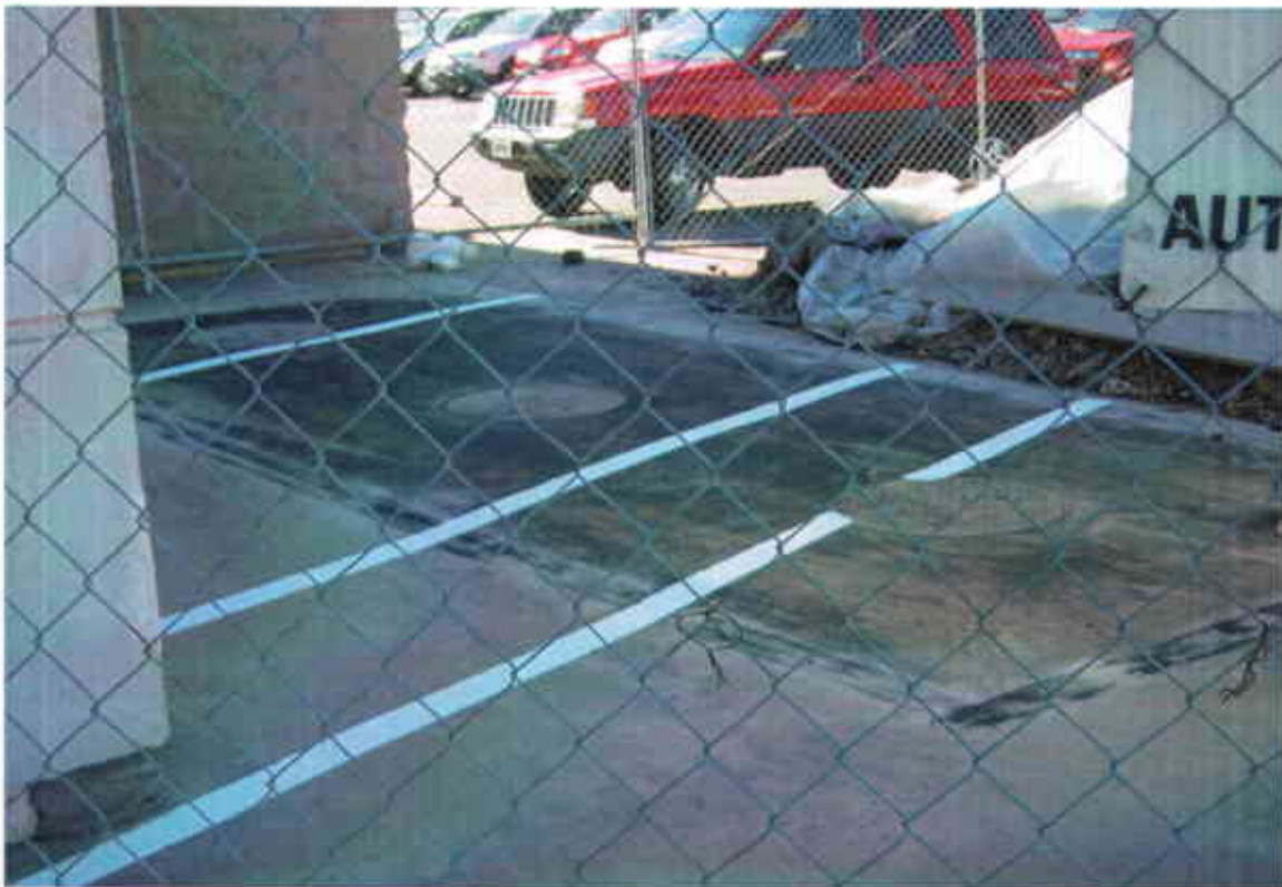
Photo #12: View of the OWS location following the completion of surface restoration.
