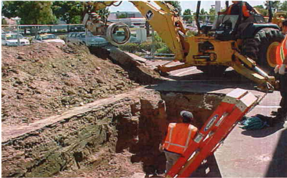
Photo #3: View of excavated soils being temporarily staged adjacent to the OWS location.
