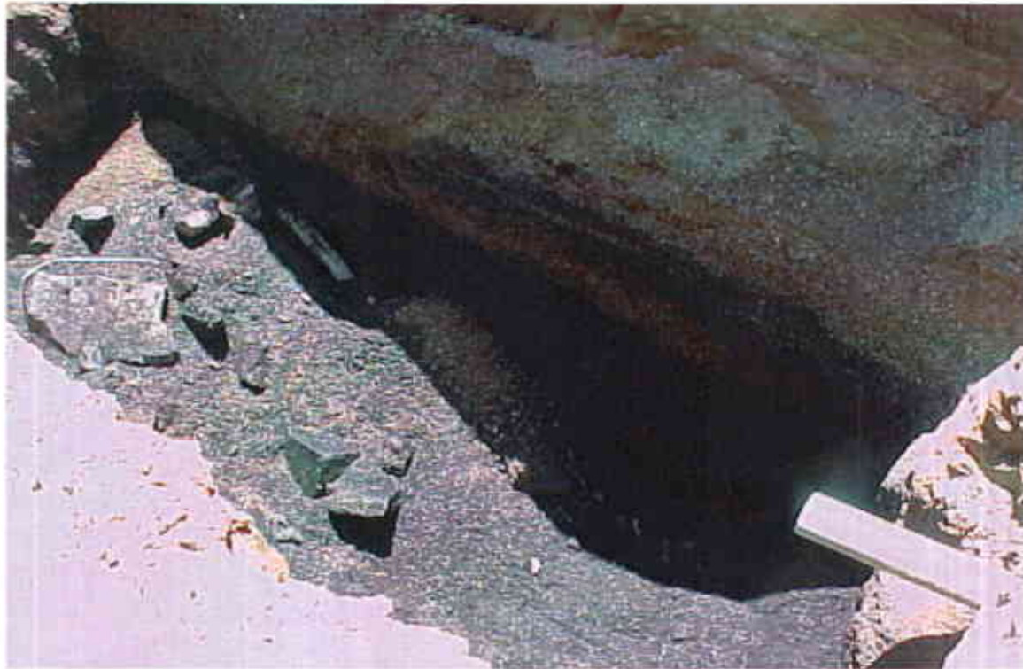
Photo #5: View of the OWS excavation following the removal of the existing OWS.
