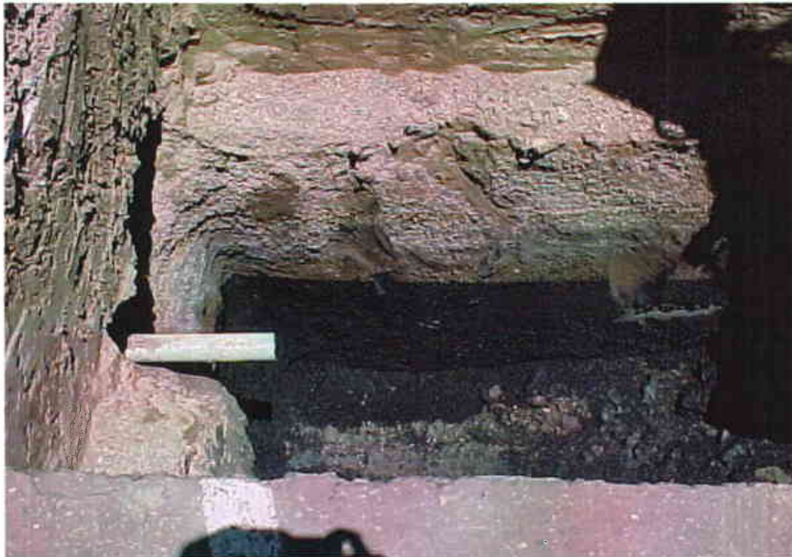
Photo #4: View of the OWS excavation following the removal of the existing OWS.
