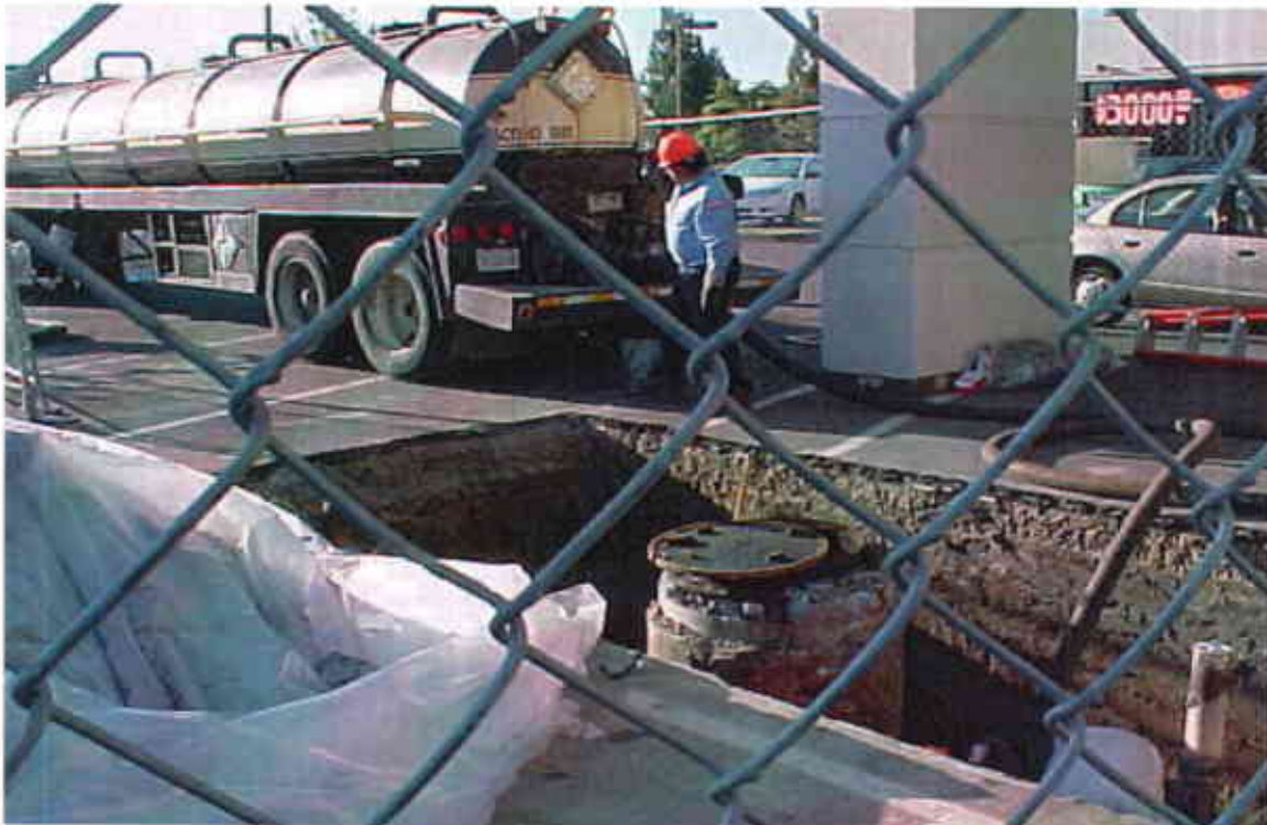
Photo #2: View of liquids being removed from the existing OWS for off Site disposal.
