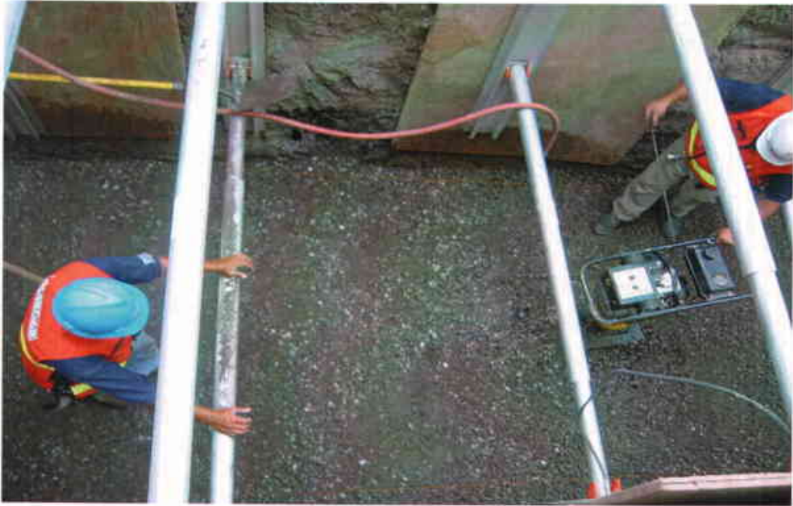
Photo #7: View of the placement and compaction of gravel bedding in the OWS excavation.
