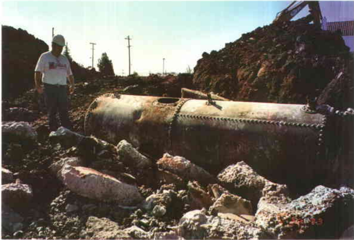
Plate 16: Tank No. 3 Shown After Concrete Casing Was Removed Note: Obsolescent design of tank and riveted plate construction.
