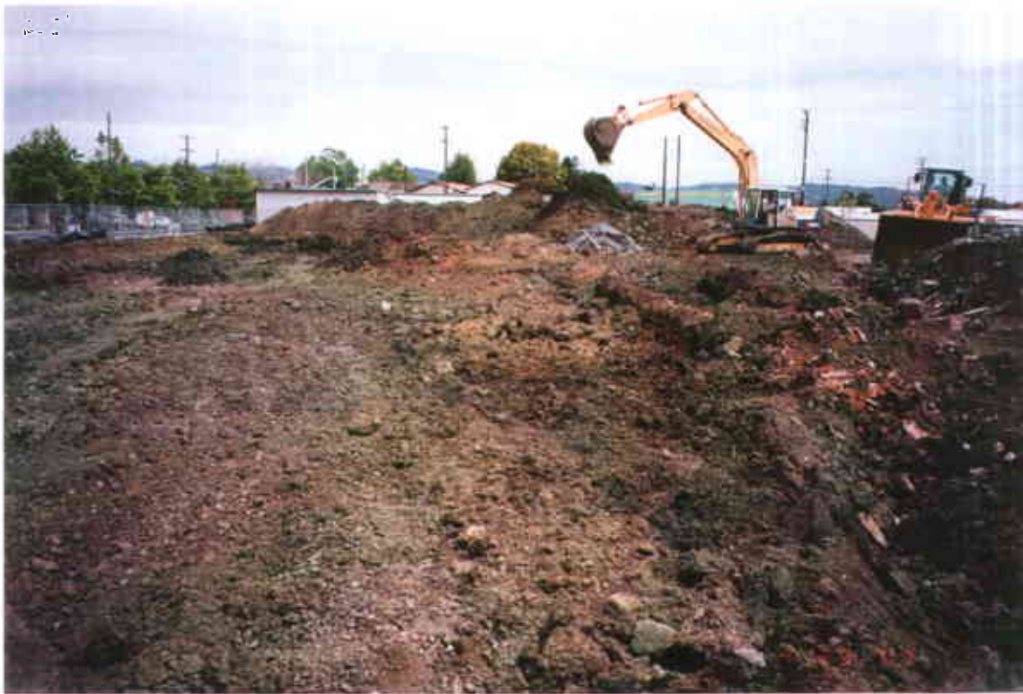
Plate 3: Clearing Clean Surficial Soil from Remediated Area Note: Clean soil stockpile is seen in background
