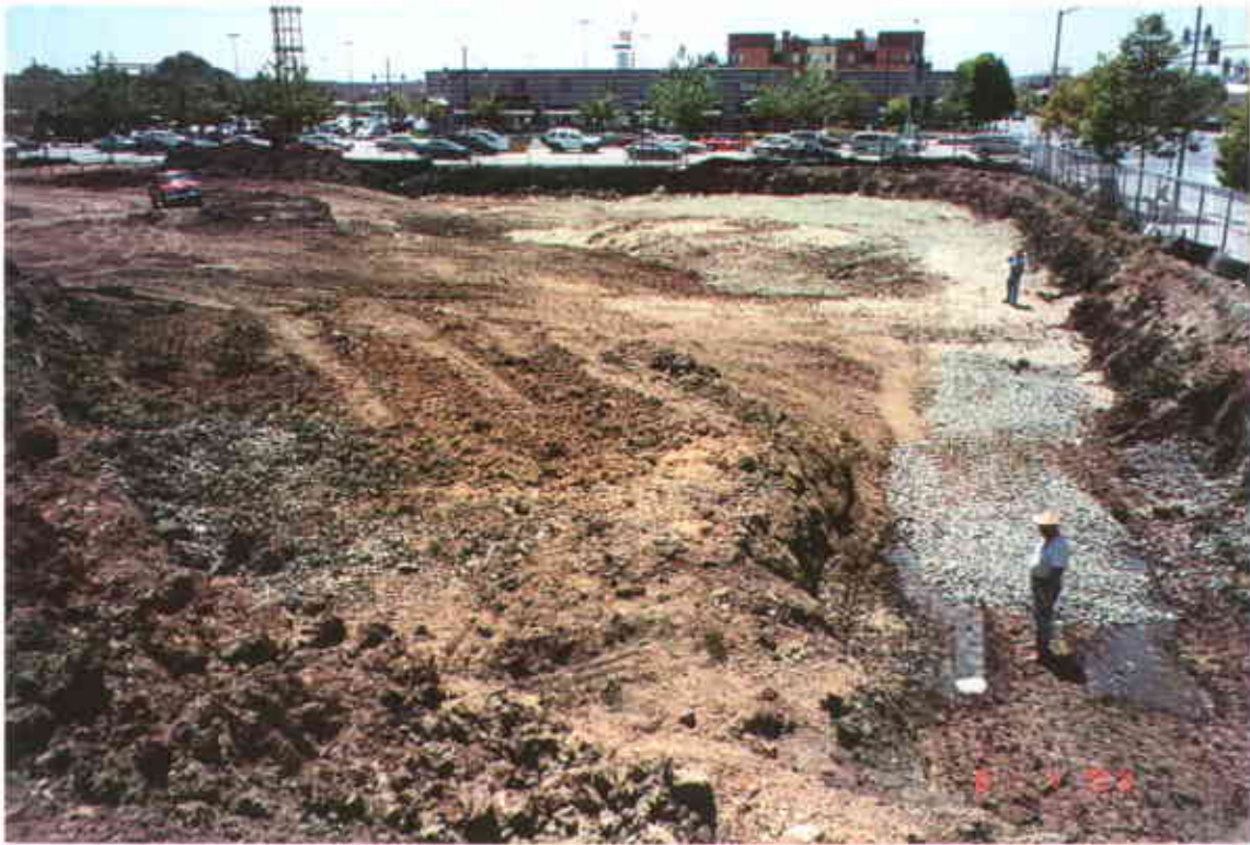
Plate 13: The Remedial Excavation Viewed from the East Note: Gravel fill is located in areas where excavation extended below the water table.
