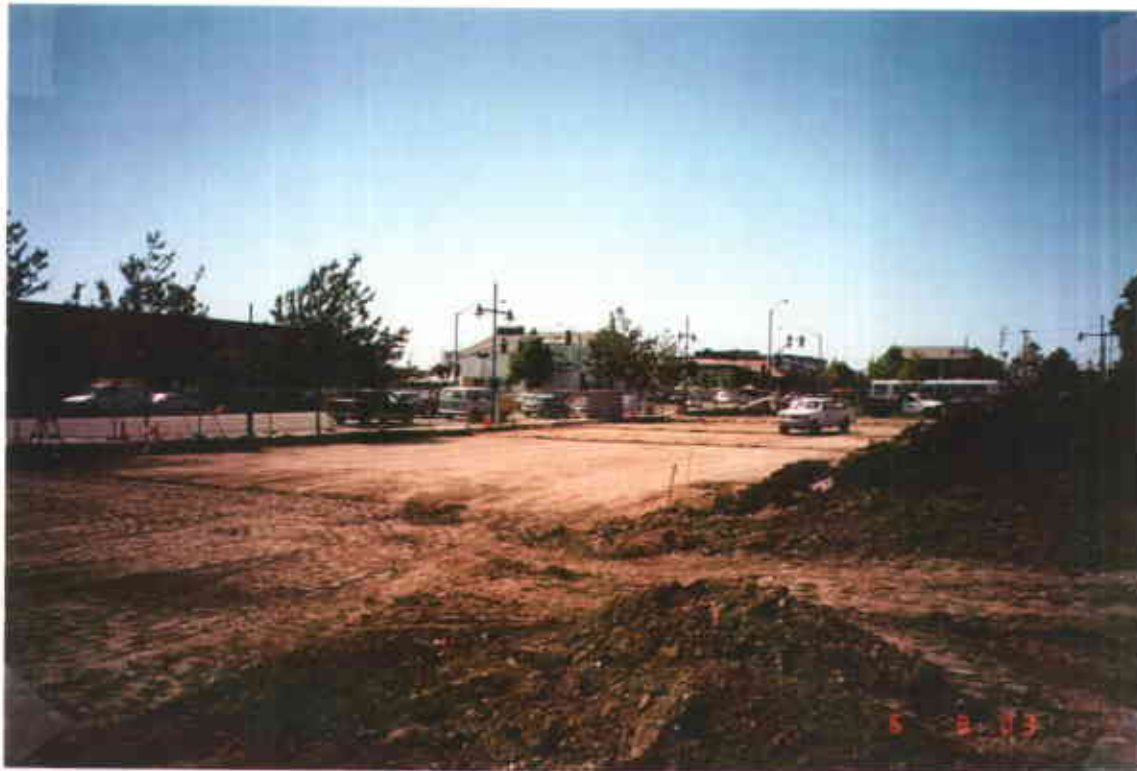
Plate 17: Western Portion of Remediation Backfilled to Grade Note: Soil for backfilling is seen stockpiled in right of photograph.
