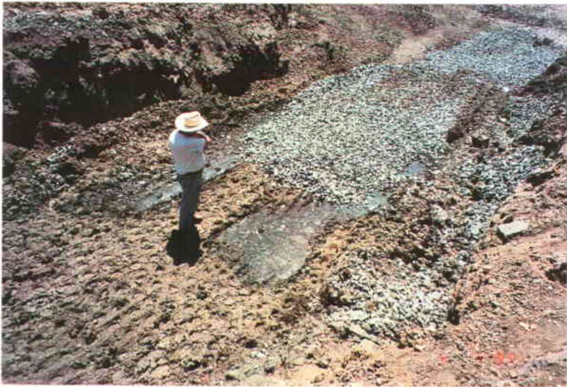
Plate 12: Transition between Backfilled Paleo Stream Channel and Clay Plug Note: Engineer is standing on clay in plug compacted by vibratory sheep's-foot compactor.
