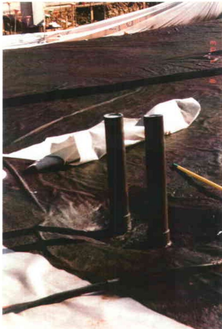
Plate 20: Membrane Seal Around Utility Duct Passing Through Floor Slab of Building 1
