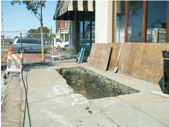
PHOTO 1: UST EXCAVATION CAVITY PRIOR TO REMOVAL, LOOKING WEST TOWARDS SAN PABLO AVENUE.
