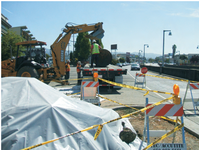
PHOTO 3: LOADING UST ONTO FLATBED TRUCK. SOIL STOCKPILE IS ON LOWER LEFT SIDE OF PHOTO.
