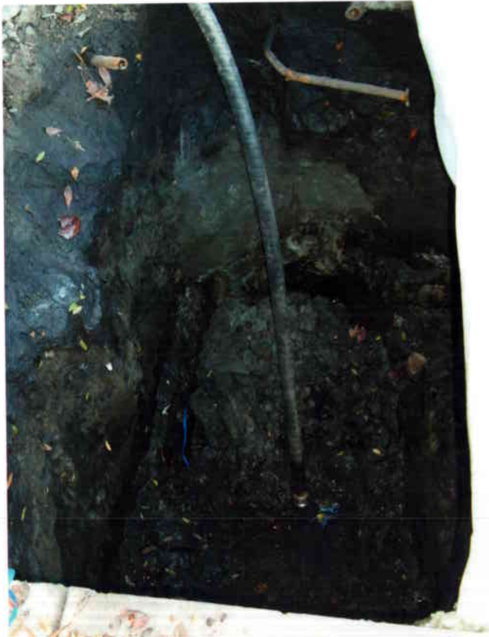
2515 Blanding Avenue Alameda, CA 94501 January 3, 2003 excavation pumped out by vacuum truck 1000 gallons of water removed
