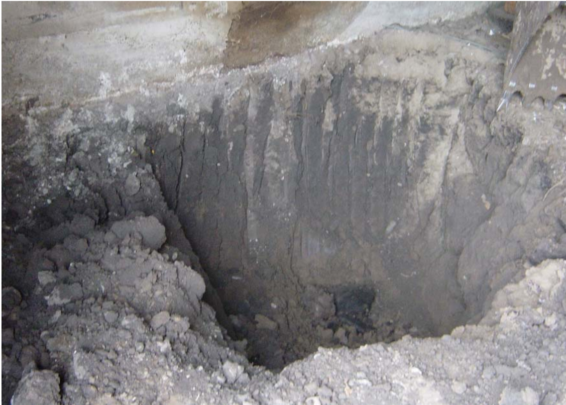
Photo 1. Close-up photo showing area beneath the former AST during excavation on March 25, 2004
