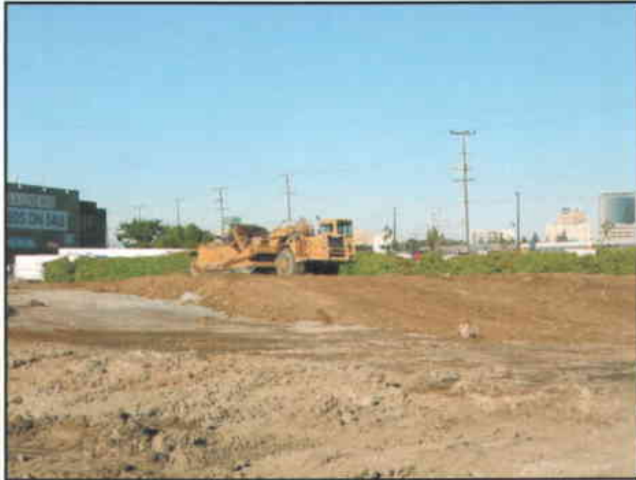
Photo #19: The sand and soil fill from the Building 1 foundation were mixed and used during mass grading of the Site.
