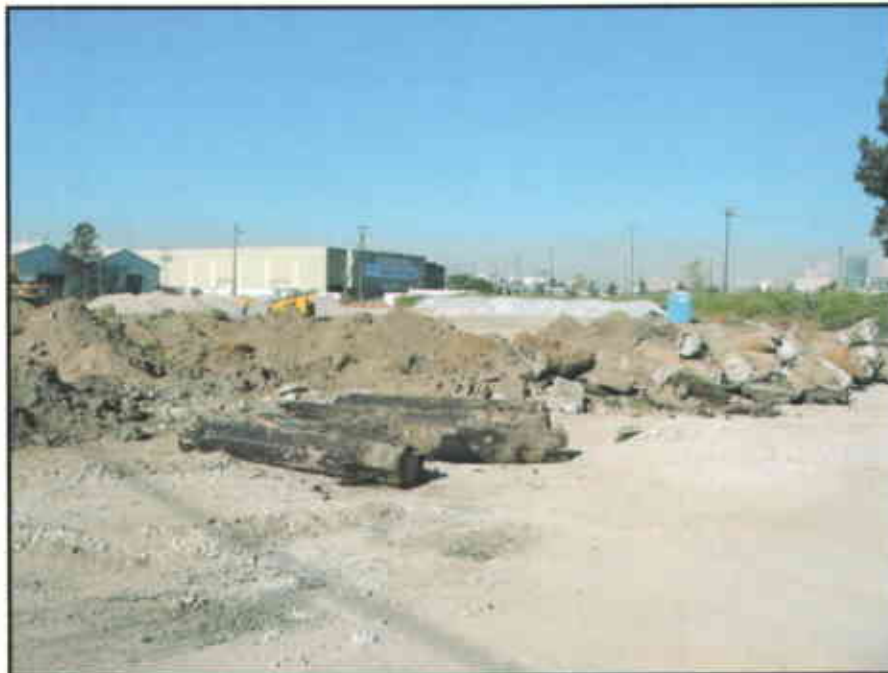
Photo #12: Timber and composite foundation piles were removed to a depth of approximately five feet below the surrounding ground surface.
