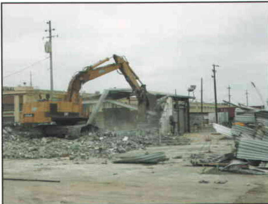
Photo #4: Demolition of concrete masonry walls and removal of steel roof girders from Building 2.
