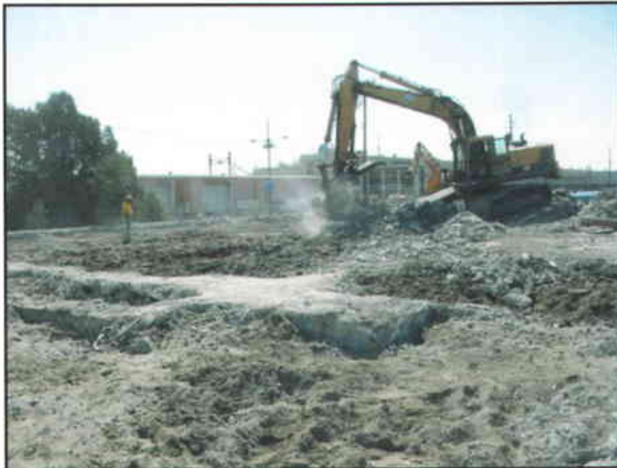
Photo #6: Demolition of Building 1 foundation revealed internal concrete shear walls and abovegrade sand and soil fill.
