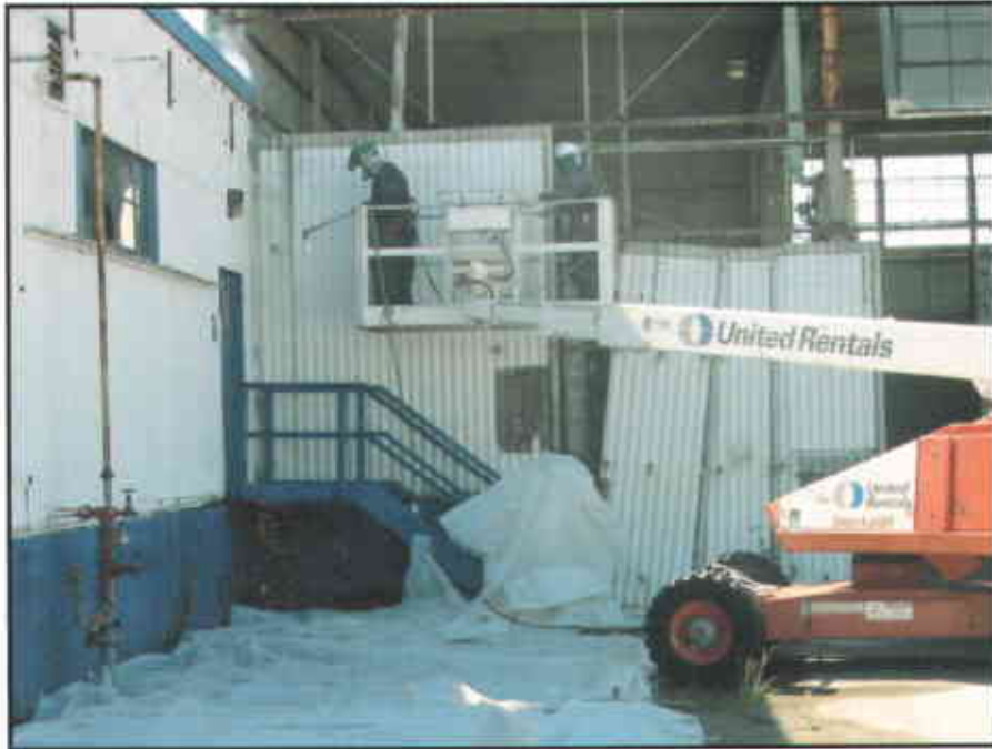
Photo #3: Transite siding was removed from Building 1 during asbestos abatement prior to demolition activities.
