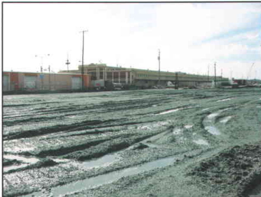
Photo #20: The Site following final grading activities. Note placement of silt fence along west and south edge of the Site and hydroseeding on disturbed soil surfaces (green tint).
