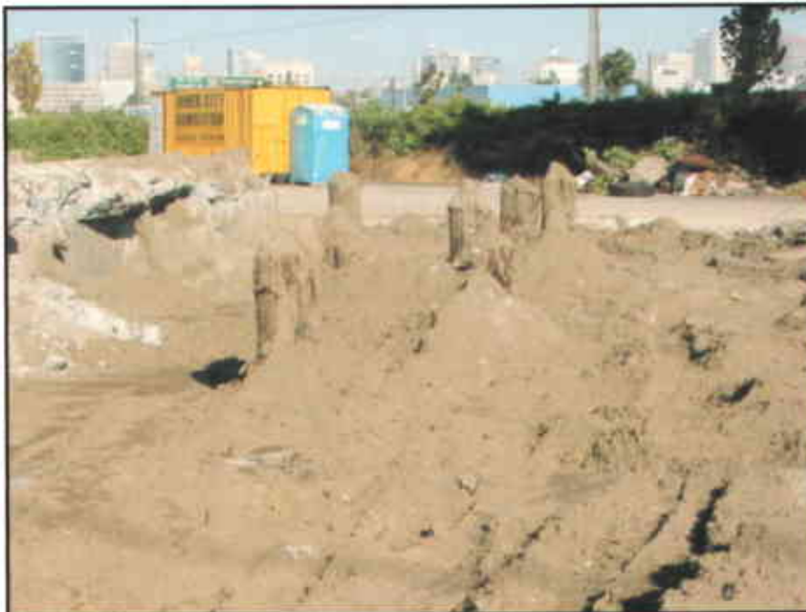
Photo #10: Timber foundation piles exposed following excavation of Building 1 foundation sand fill.
