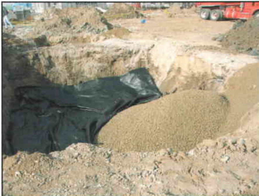
Photo #16: Mirafi fabric and drain rock were used during backfilling in areas where soft, plastic native soil were exposed.
