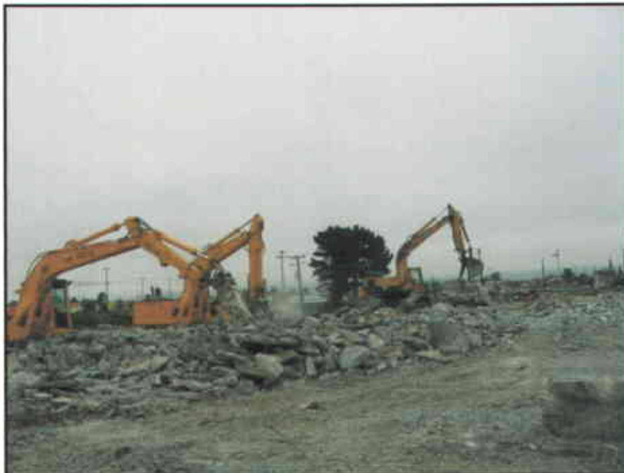
Photo #14: Demolition debris was processed by crushing concrete, removing steel reinforcement, and off hauling to appropriate recycling facilities.
