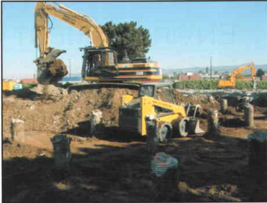
Photo #9: Building 1 foundation soil fill was excavated to expose composite foundation piles.
