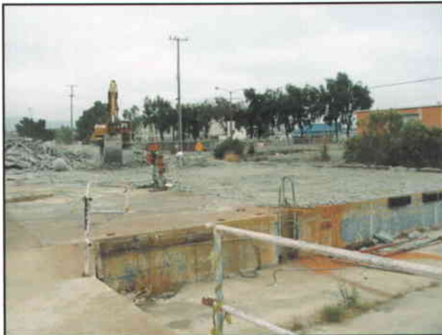
Photo #8: The Building 2 foundation consisted of a concrete slab on grade, which was demolished using an excavator.
