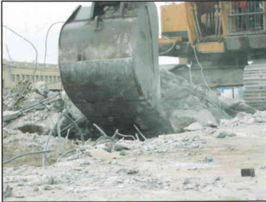
Photo #5: Demolition of Building 1 foundation. Note thickness of concrete, large diameter of rebar, and abundance of rebar.
