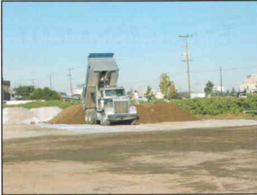
Photo #11: Sand and soil fill from the Building 1 foundation was stockpiled along the northern portion of the Site.
