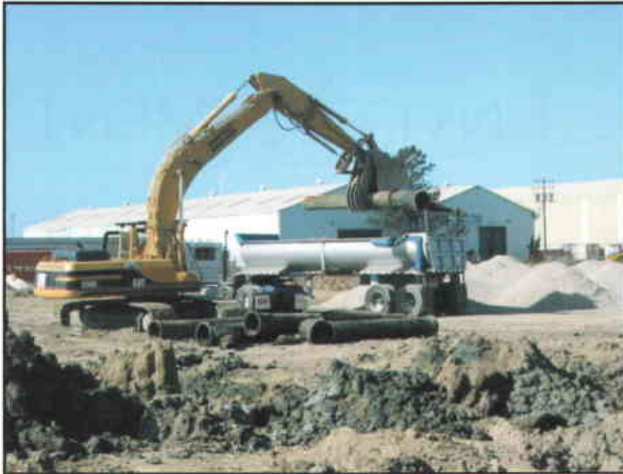
Photo #15: Process and utility pipelines were excavated and removed from the Site.
