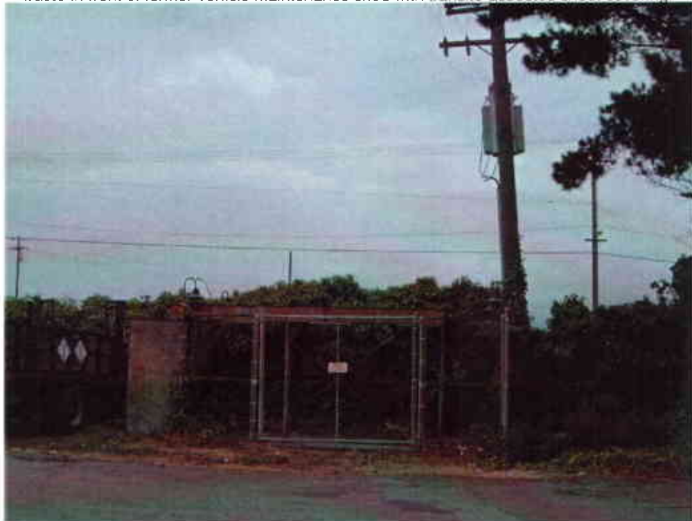
Photo #4: View looking north at former PG&E transformers slab and cage, replaced with pole-mounted transformer (upper right) following June 2000 transformer failure. Utility meter within metal cabinet, left of slab/cage
