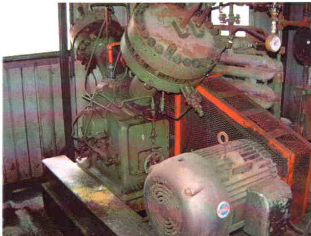
Photo #11: View of thrown oil and absorbent (yellow when wet) next to leaking piston compressor in attached room on northwest side of Building One.
