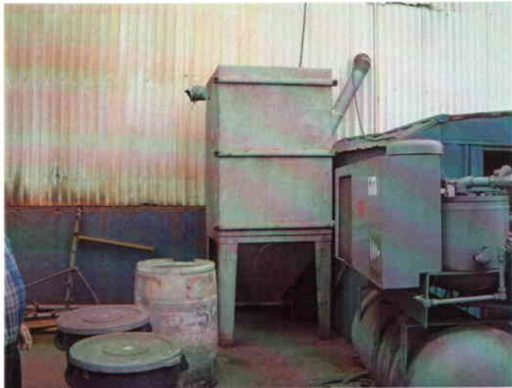
Photo #5: View looking southeast at paint-dust containment bin from bead blast (inside) on northwest side of Building One. Bottom emptying bin too short to directly fill drums. Three containers in left foreground (two garbage cans are full, uncovered drum two-thirds full) are unlabeled.
