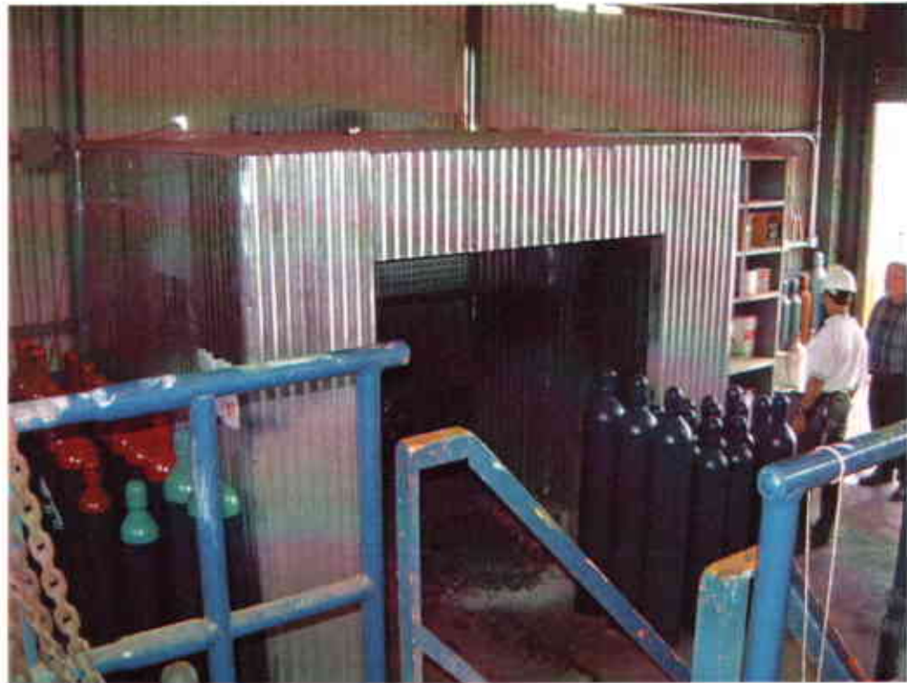
Photo #9: Newly constructed paint booth along southwestern wall of Building One. Paint spray booth permit with Bay Area Air Quality District was pending at time of reconnaissance.
