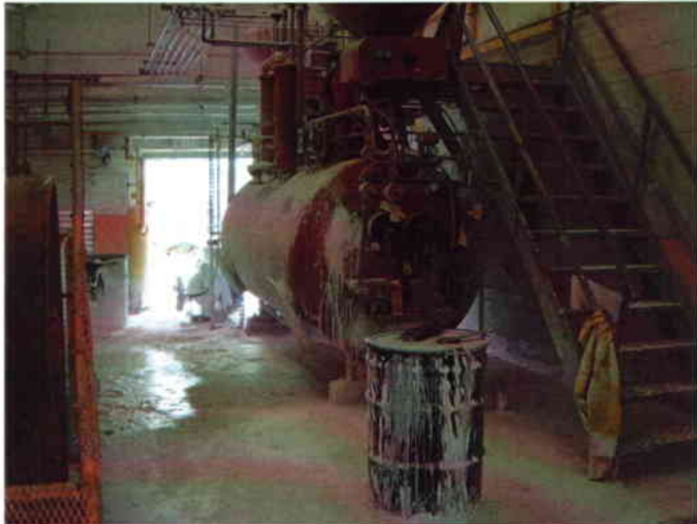
Photo #14: View looking north inside acetylene reactor room in Building Two. Note carbide lime spillage on floor.
