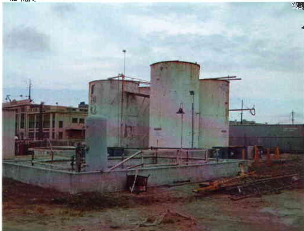
Photo #16: View looking south at high pH water pit with four, water/carbide lime settling tanks behind. Port of Oakland 9 th Avenue Terminal in left background.
