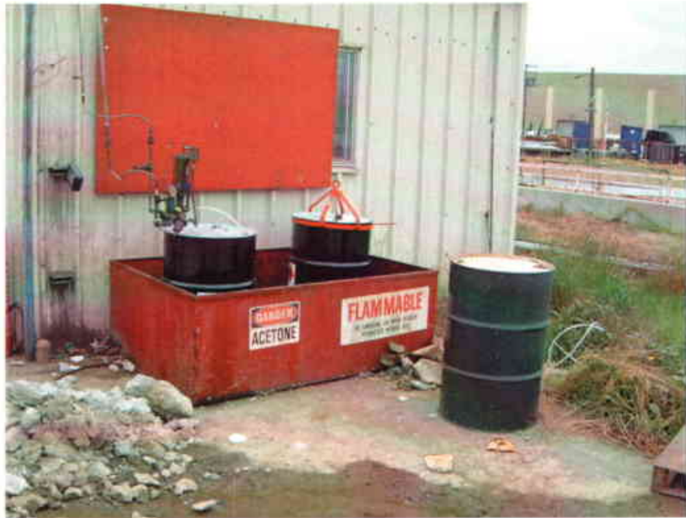
Photo #17: Acetone drums in uncovered metal containment bin on east side of storage shed north of Building Two. Full acetone drum outside of containment bin. Note corroded metal base of bin and proximity to bare ground. Liquid in foreground from leaking water pipeline
