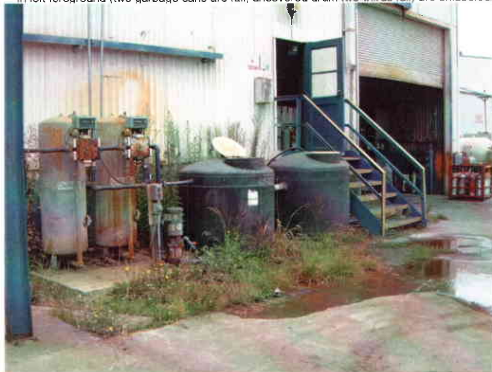
Photo #6: View looking at leaking hydrostatic cylinder testing sump water outside north wall at southern end of Building One. Spilled water in right foreground flows short distance to storm drain drop inlet, then drains to bay.
