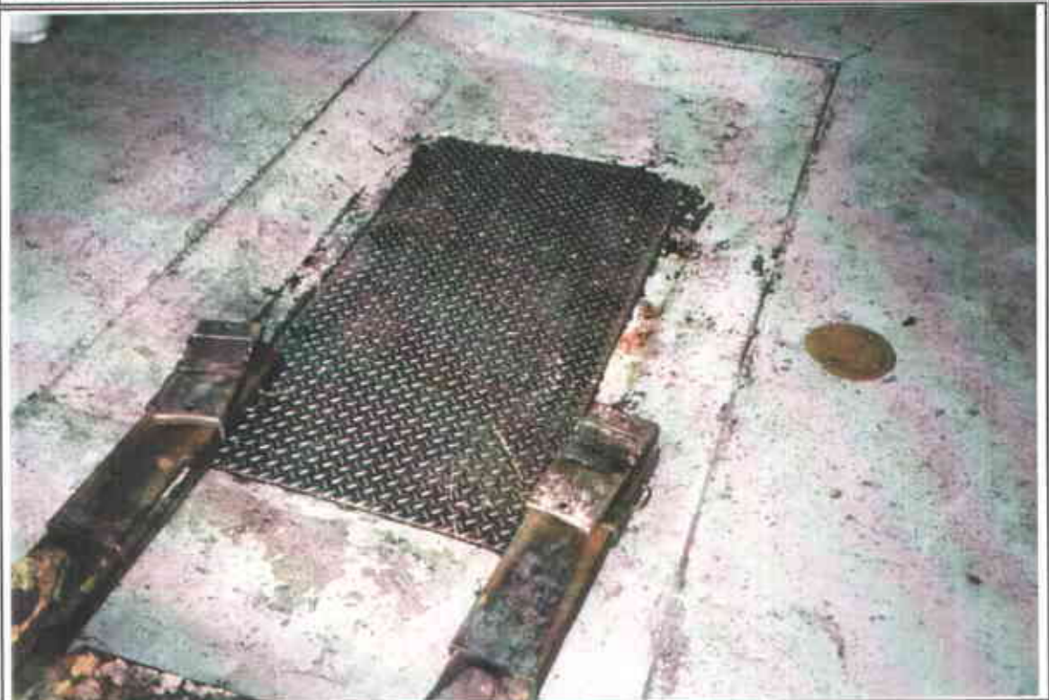
Photograph 6: View of the car hoist and the sealed oil and grease separator inside the repair shop.
