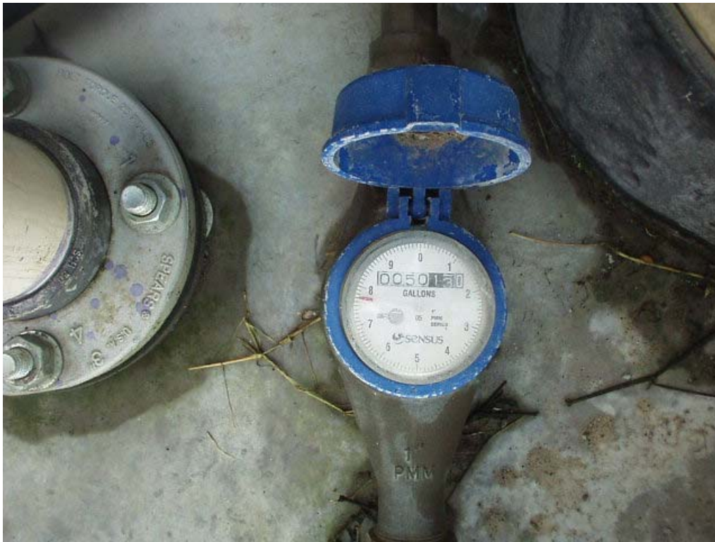
010-Outside Flow Meter.jpg
