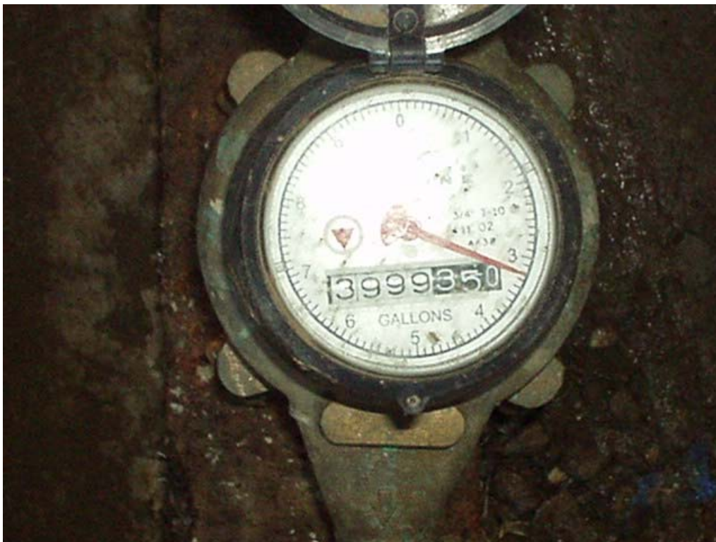
009-Inside Flow Meter.jpg
