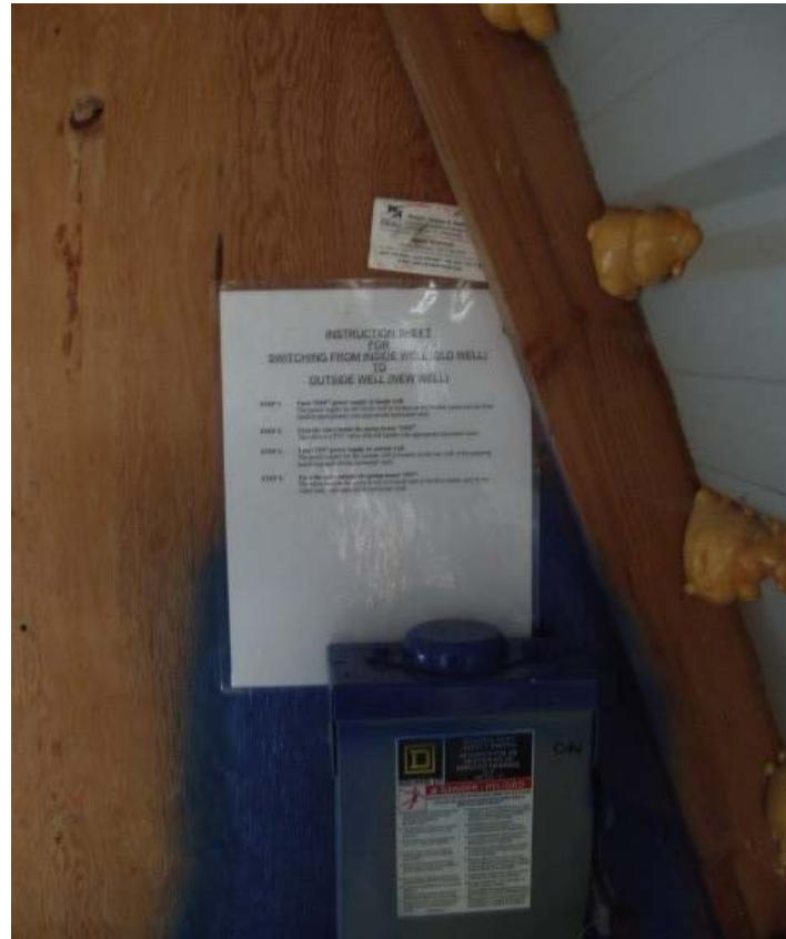
Outside Well Power Switch.jpg
