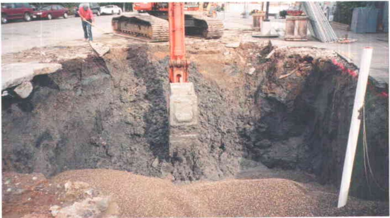
View showing the backfilling of the UST excavation cavity with clean imported gravel in foreground, while overexcavation continues at other end of excavation cavity. Note standpipe well on right side of photo.
