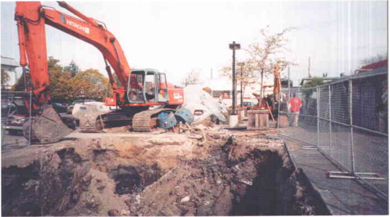
View of UST removal area. Note covered excavated soil stockpile in middle of photo and dispenser island to right of stockpile.
