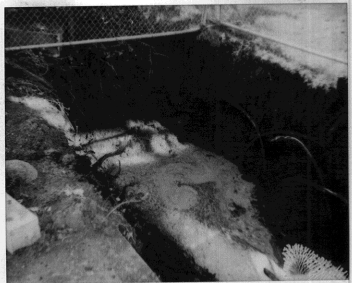
10-21-94 water in 3000 gal UST pit
