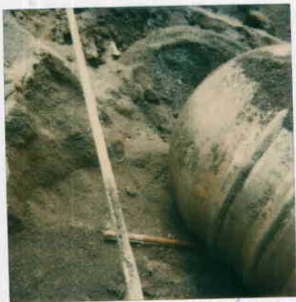
South end of unleaded fuel tank. 15526 Hesperian Blvd., San Lorenzo Chevron 5-30-91
