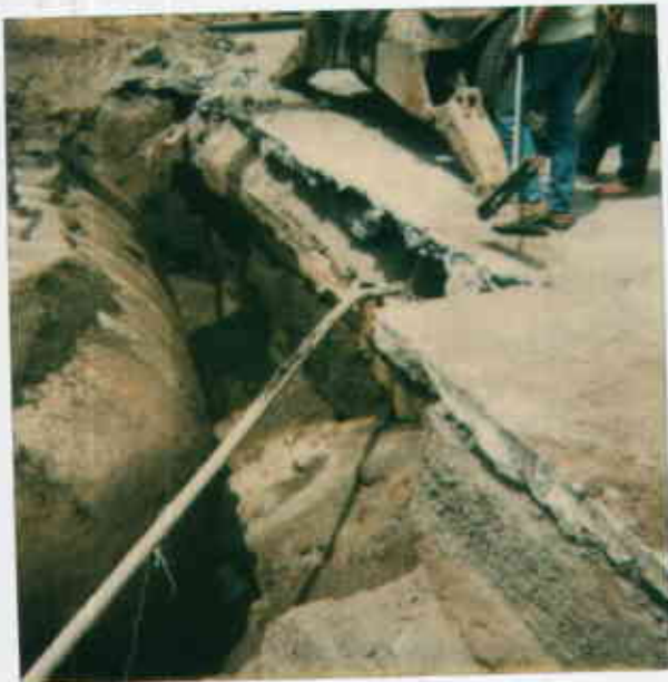
Unleaded tank - dark soil appears stained. 15526 Hesperian Blvd, San Lorenzo. Chevron. 5-30-91
