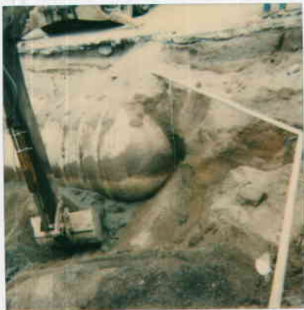
Unleaded tank - dark soil appears stained. 15526 Hesperian Blvd Chevron, San Lorenzo. 5-30-91
