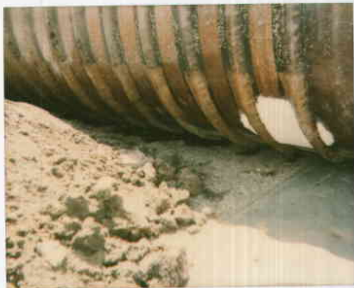
Supreme Unleaded Tank - liquid puddling (dark area) beneath tank. 15526 Hesperian Blvd, San Lorenzo - Chevron 5-30-91
