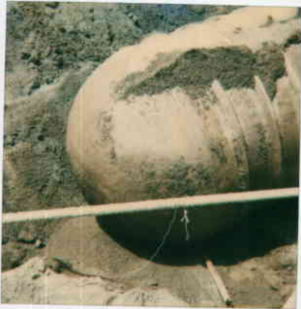
Unleaded fuel tank - 15526 Hesperian Blvd, San Lorenzo 5-30-91. South end of tank
