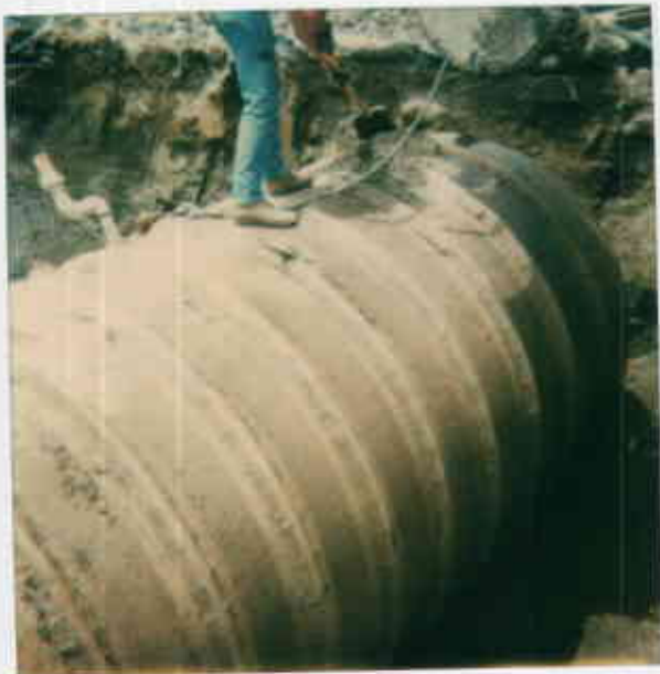
Unleaded tank - spurge beneath workers foot. 15526, Hesperian Blvd, San Lorenzo. Chevron 5-30-91
