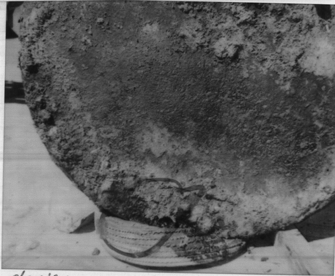
8/30/95 3623 Adeline (hole at bottom at the end of the tank pipes)
