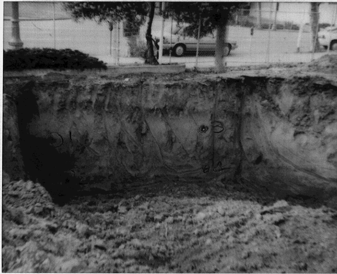
Front pit spilling @ 460 Grand Ave 1/20/94
