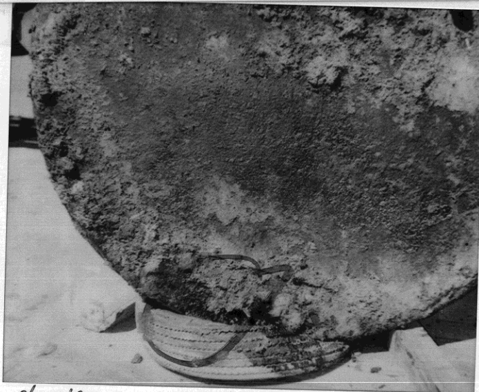
8/30/95 3623 Adeline (hole at bottom North end of the tank pipe connected to PLS)
