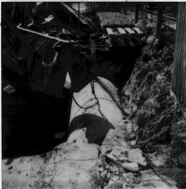
FILL PIPE VISIBLE AT SOUTH END OF TANK
