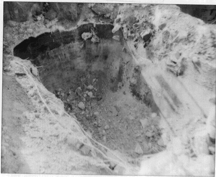
Rotten concrete vault 4701 57/12 San Carlos & G. Wood
