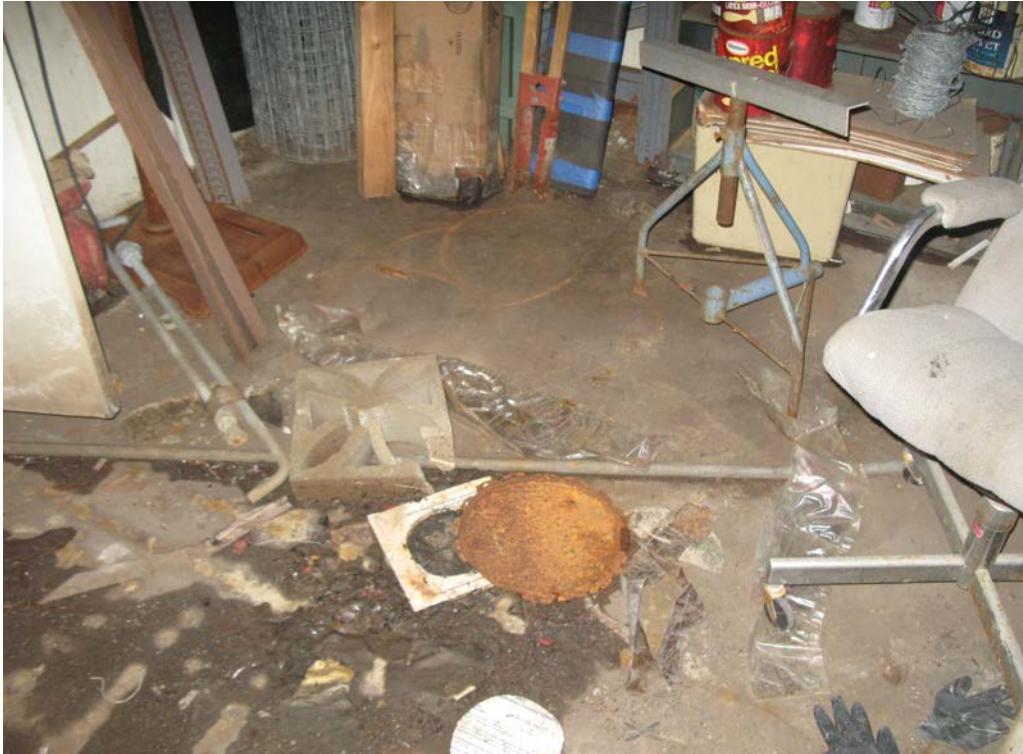
Photo 9: Floor of maintenance area in warehouse building. Floor staining appeared to have been caused by water intrusion.
