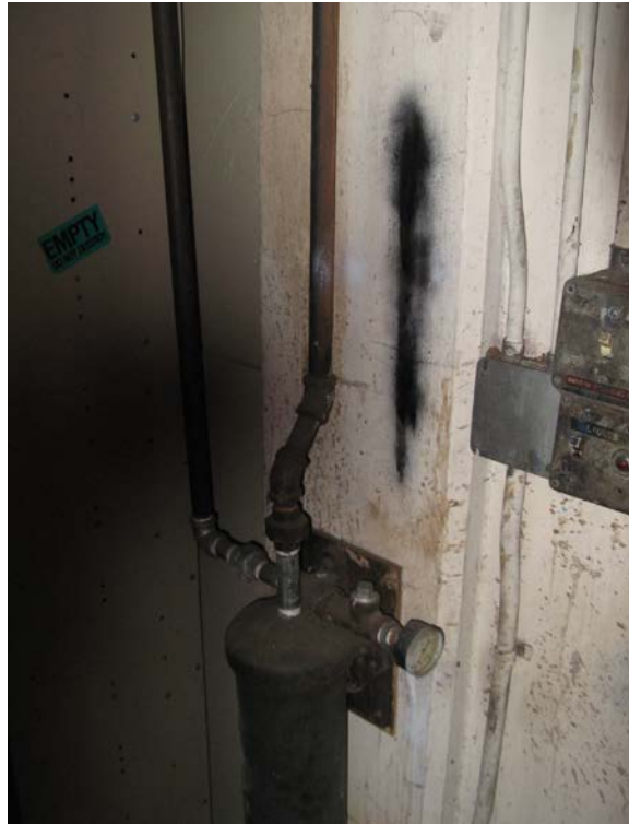
Photo 15: Hydraulic system equipment in unused area of warehouse building.
