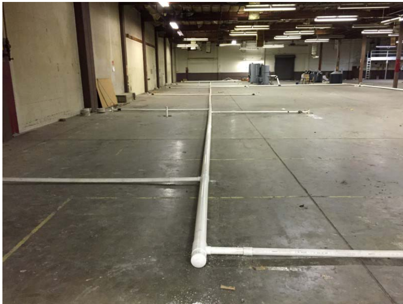
Photo 2. View of SVE well piping and central collection piping. SVE system visible in distance.
