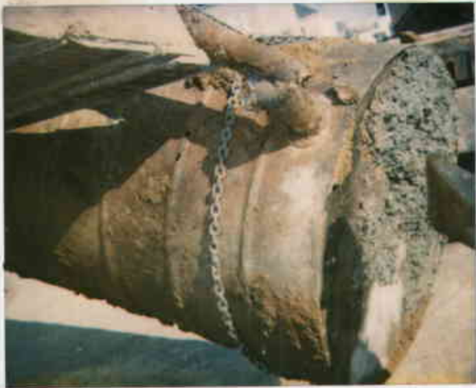
Holes on north fill end of Tank #2 1/19/94 1200 20th Ave Cholera-densum also
