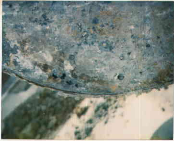
South end of Tank #2, Seam has corroded through 1/19/94 1200 20th Ave
