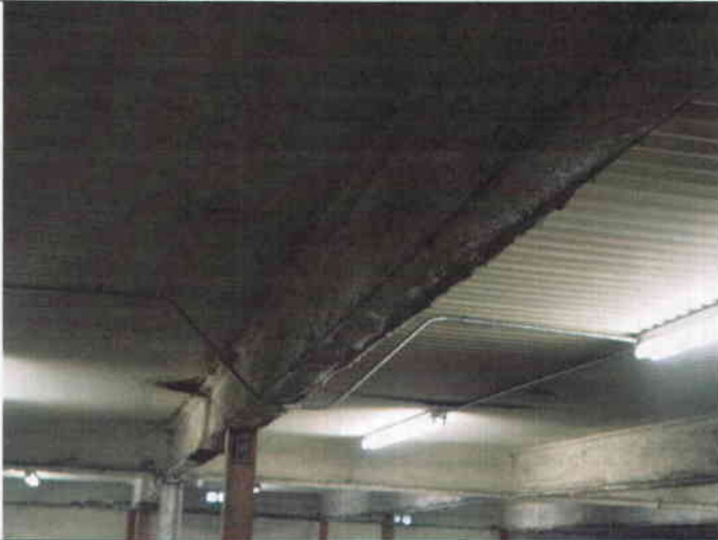
Sprayed-on fireproofing in parking basement
