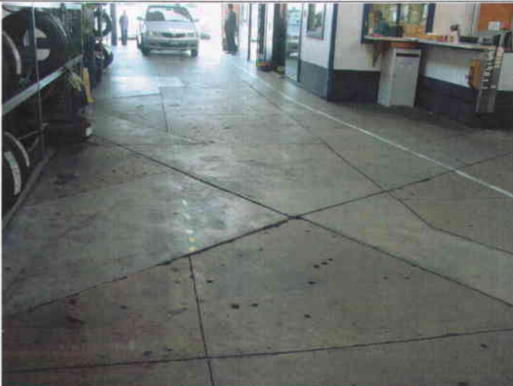
Concrete patches in floor at former car wash (3735-37)
