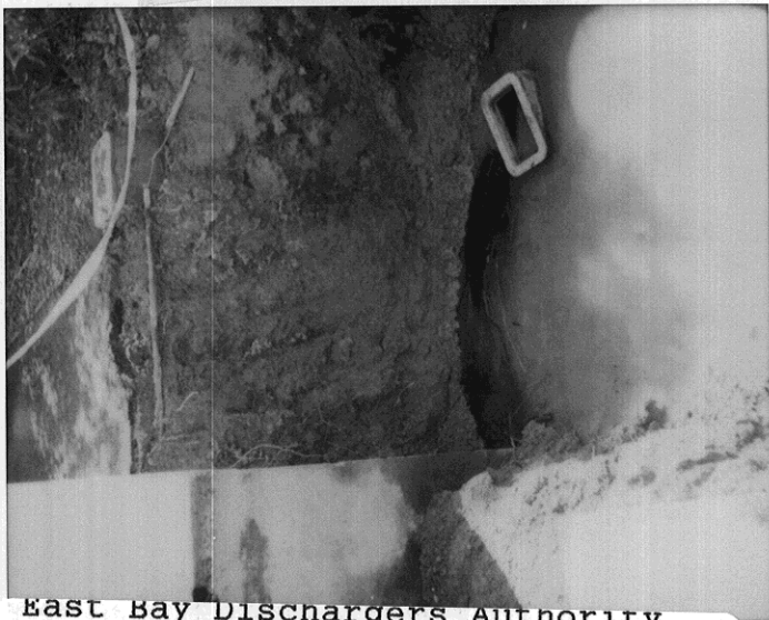
East Bay Dischargers Authority 2651 Grant Avenue San Lorenzo 2/25/99 RW Diesel fuel release FREE PRODUCT EXCAVATION TO REMOVE SOURCE
