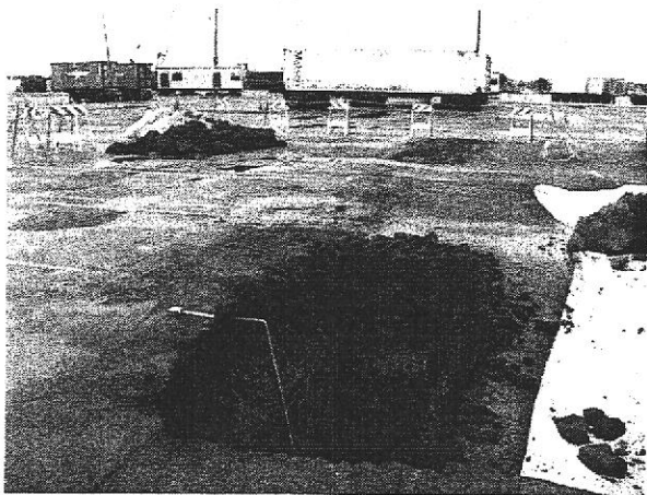
#5 Test pit TP-2. Greenish-gray clayey silt beginning at 2' bgs. Crushed rock fill and asphaltic concrete layer above. Backfilled test pit TP-1 visible in background.
