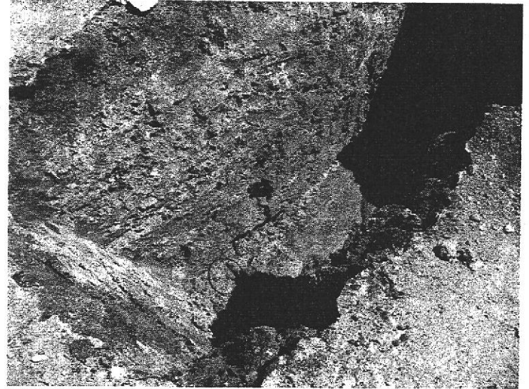
# 8 Pieces of wood debris and crushed rock visible in TP-4 northeastern sidewall down to depths of approximately 6' bgs.
