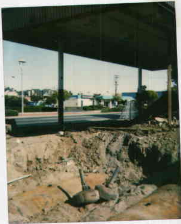
Overflow protection Basin # 604 1619 - 1st St. Livermore 03216211255-8 11/10/92
