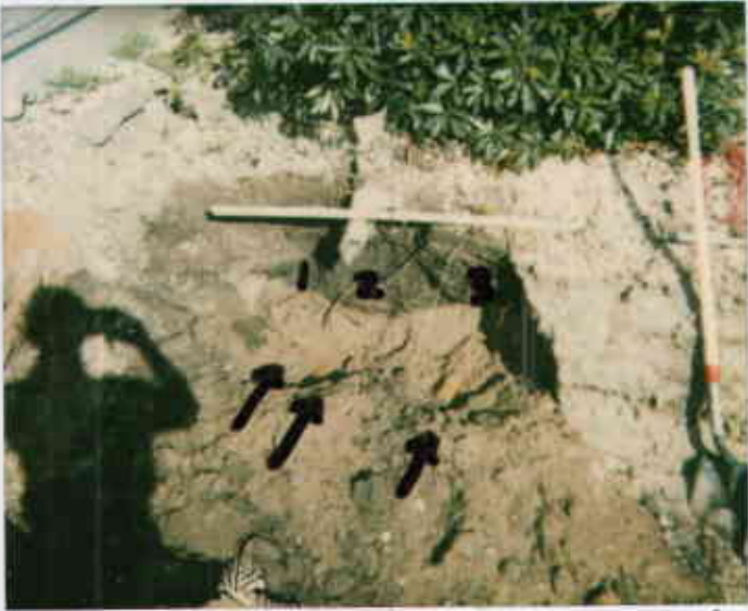
Three (3) 2" FRP product lines heading east beneath utility box (PG+E)
