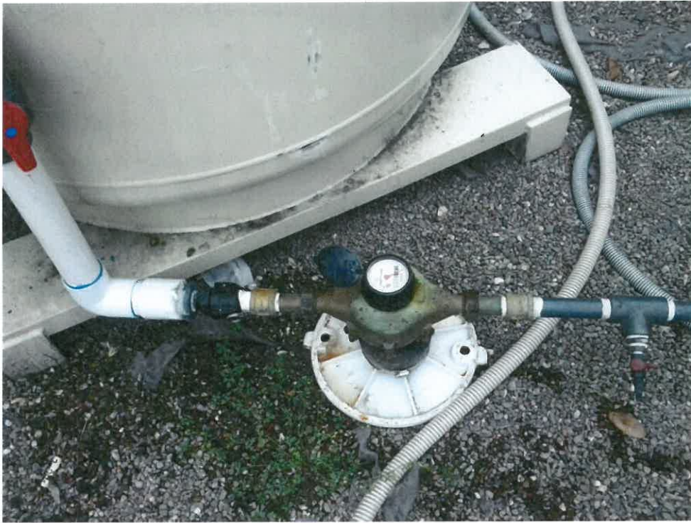
Photo 1: Standing over totalizer in revised location (after lag GAC just prior to discharge).
