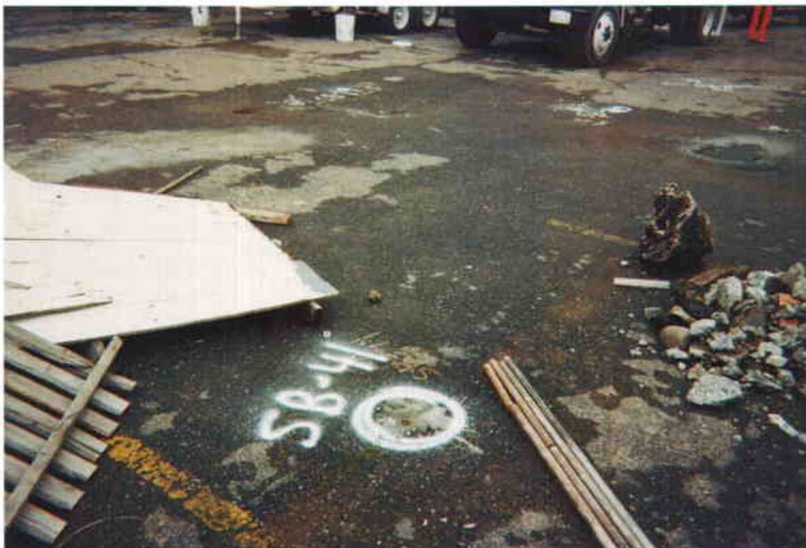
Photo 2: Soil borings along western edge of gasoline-affected soil (SB-41 in foreground and SB-19 and SB-20 in background).
