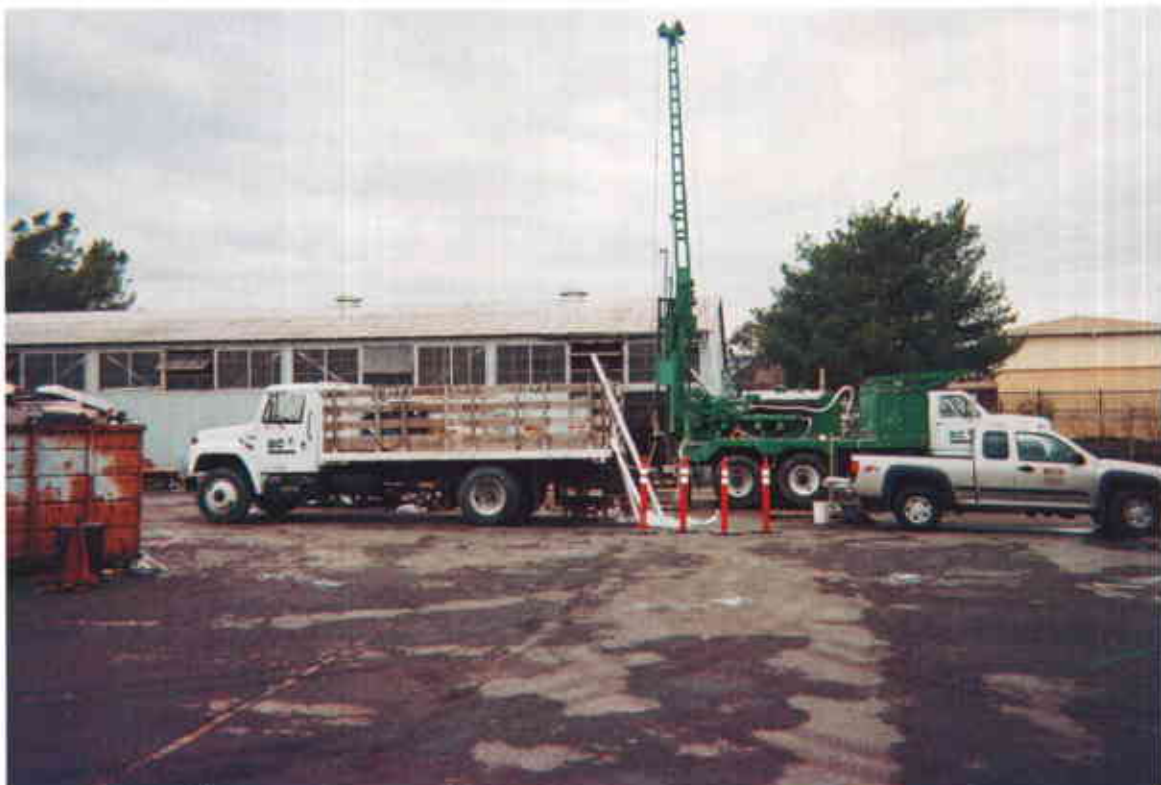
Photo 10: BC 2 Environmental drill rig and support truck during installation of nested well NW-2.
