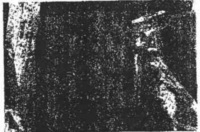
Ultra-Lite insulates steam duct to conserve energy. — Scarborough, Ontario
