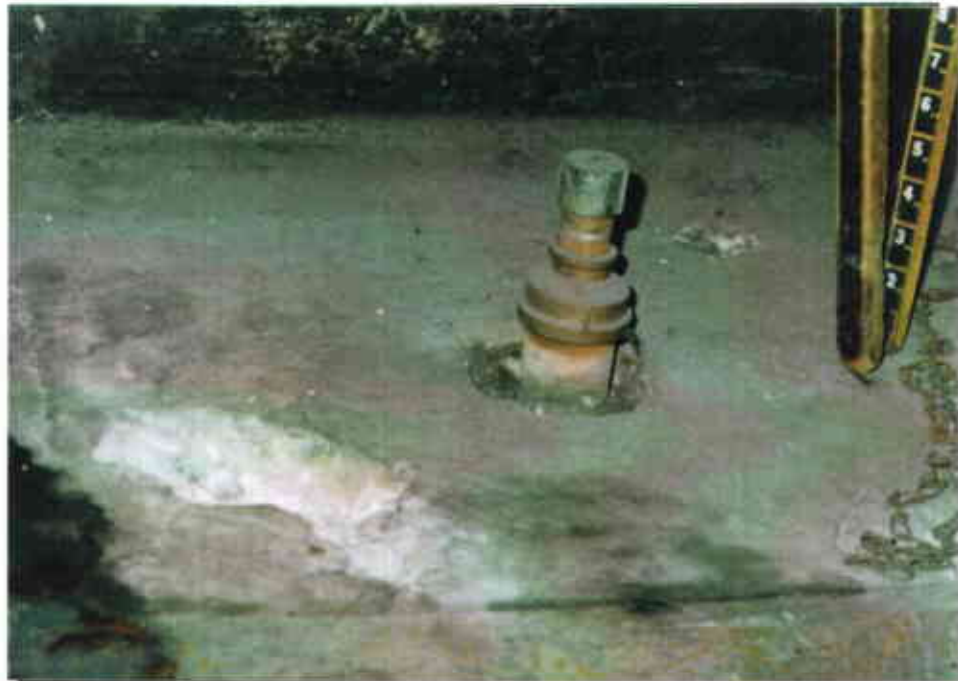
Figure 9: ALCOPARK's basement: dispenser line's riser.
