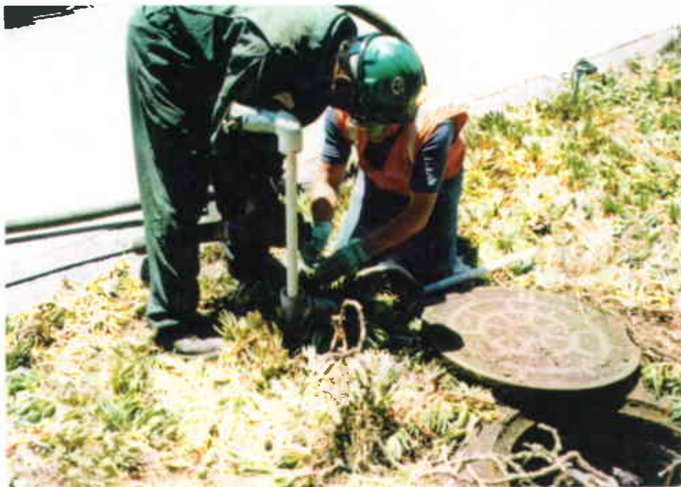
Figure 6: Sampling of rinsate from one of the USTs.
