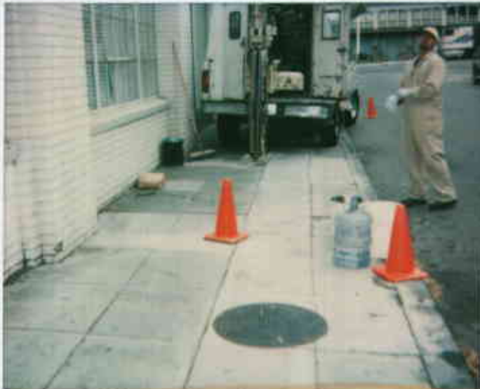
2740 Broadway, Oakland 08/05/99 Gregg Drilling at 08916310210-02 0125 5072 boring location SB-1E, located adjacent to former boring SB-3. COPIES & ENLARGEMENTS CALL 800-421-1030 - Juliet Shinn
