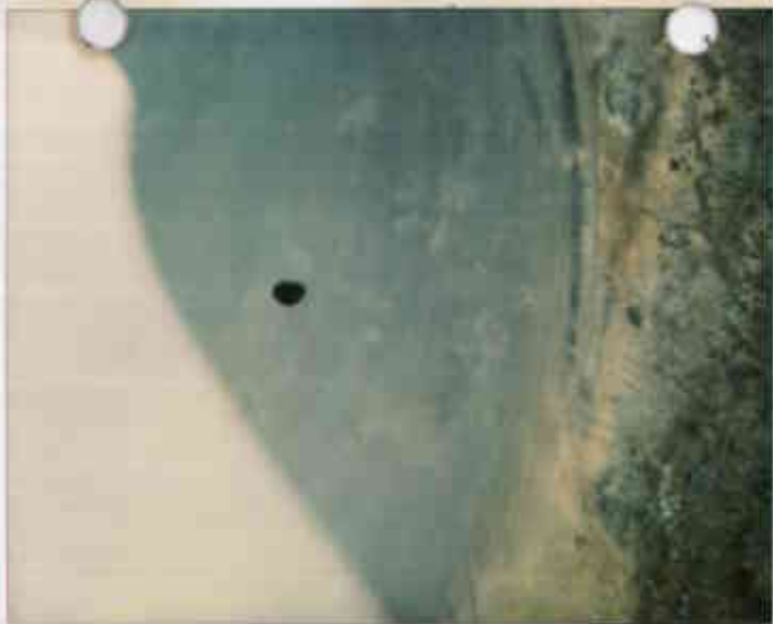
Hole, west end of Tank "A", ~3/4 y diameter 8/30/94 2549 E 276
