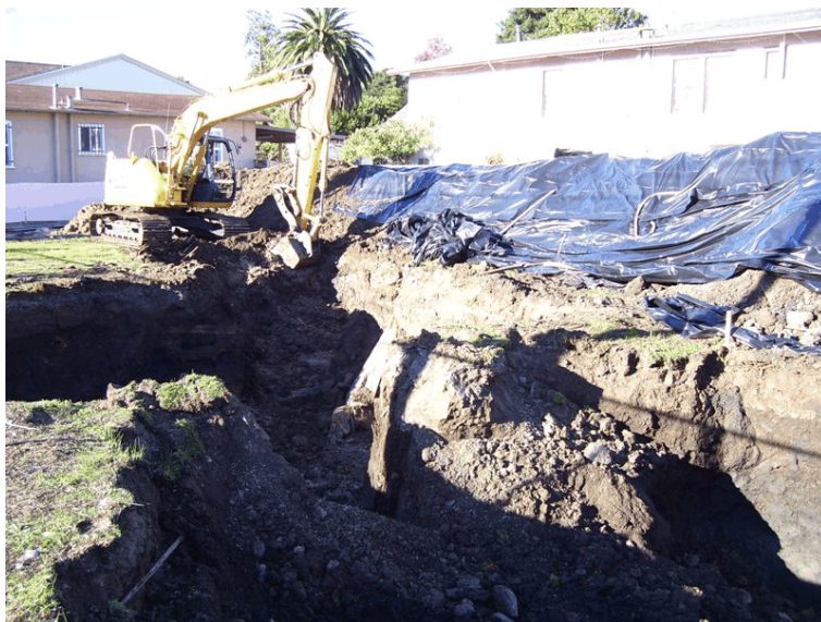
Photograph 6 - View of excavation pits, Areas I, II, and III are now connected. The excavator is working on Area III.
