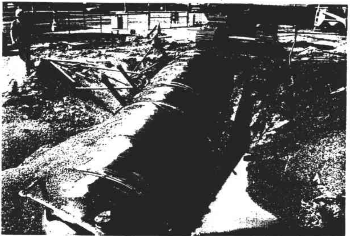
Photo 6: Tank #3 after floating to surface and dislodging concrete anchor.
