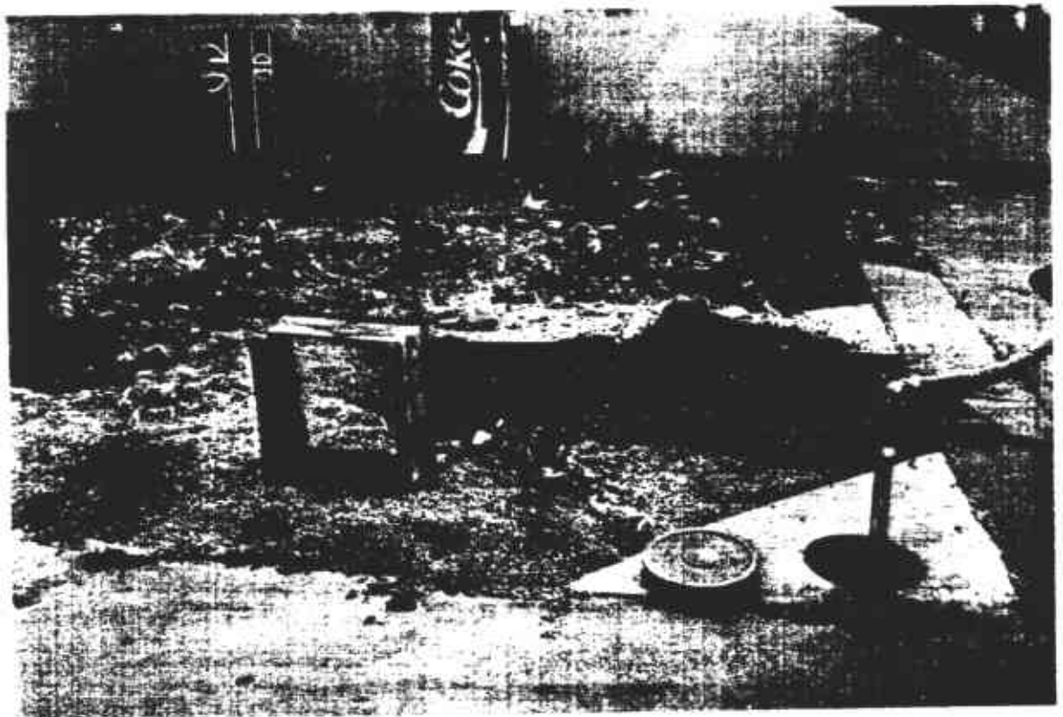
Photo 2: UST backfill material after removal of concrete slab. Pumping water from observation well in tank backfill.
