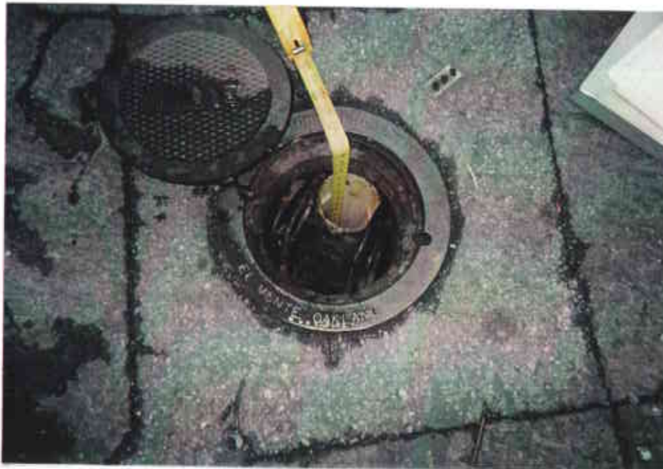
Cathodic protection well (CP1)
