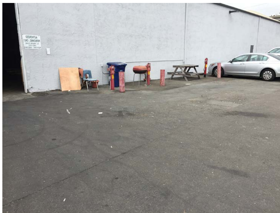
Photo #2 Warehouse fire water piping. 08/29/2017 Looking northeast
