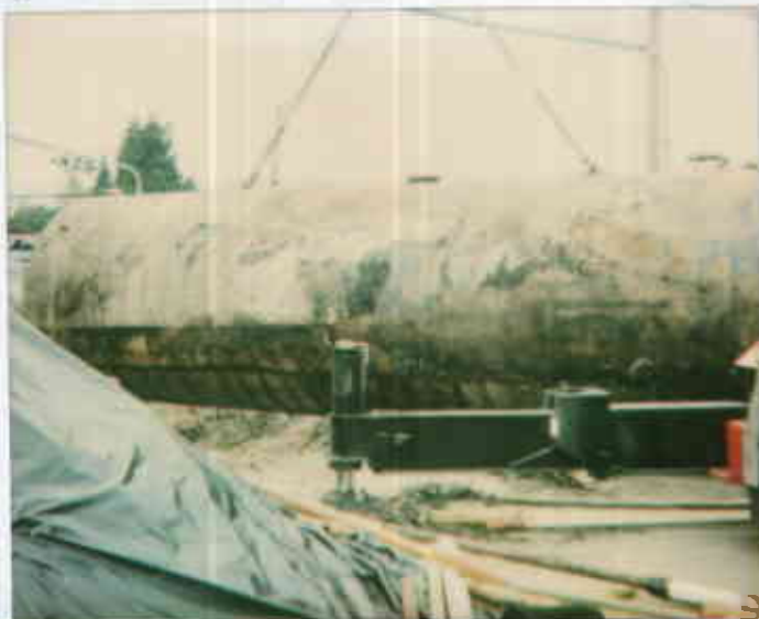
1436 Grant Ave. San Lorenzo 7/10/98 01816122077-02 1440 6588 COPIES & ENLARGEMENTS CALL 800-421-1030 10K gasoline UST - tar wrap partial dissolved around mid section
