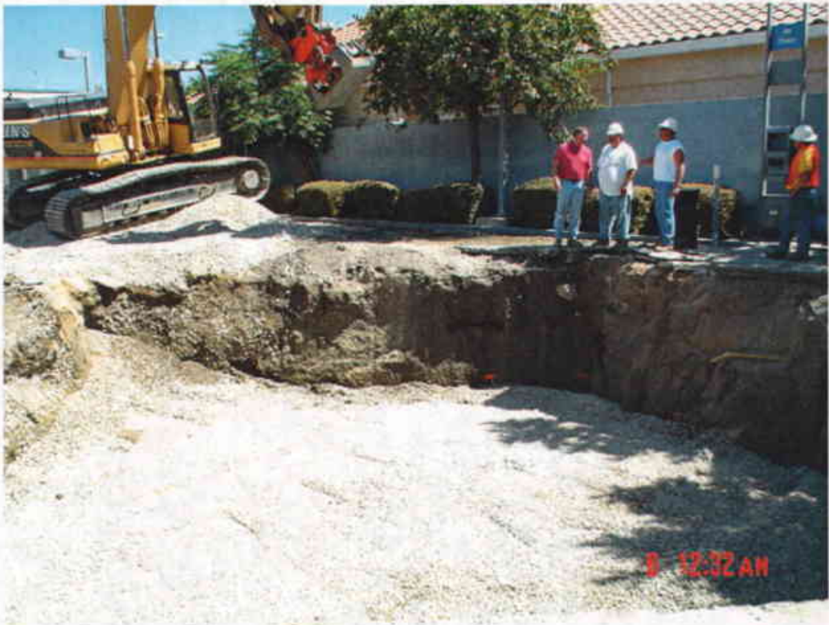
Plate 23: View Northeast showing compacted surface of drain rock performed with vibratory compactor – shown mounted on excavator.
