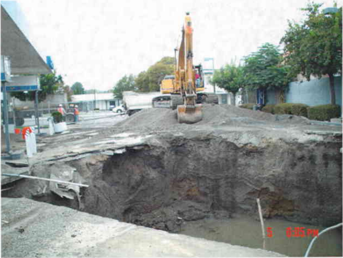
Plate 20: View North showing continued uploading of UST-pit gravel with groundwater pooled in former UST pit at approximately 11 feet bgs.
