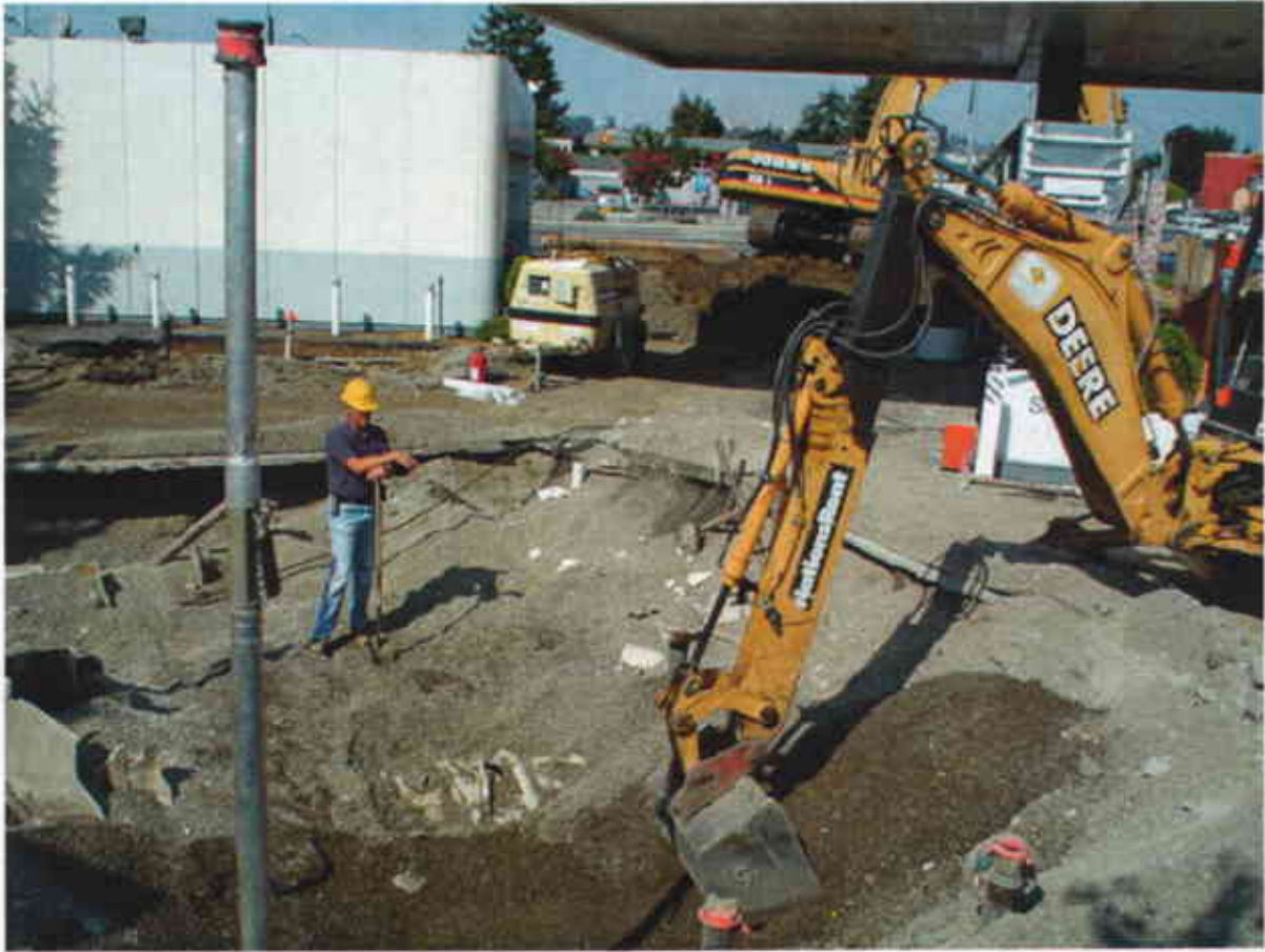
Plate 9: View to West showing continued excavation of pea gravel from existing UST pit and installed vent pipe on UST#1.
