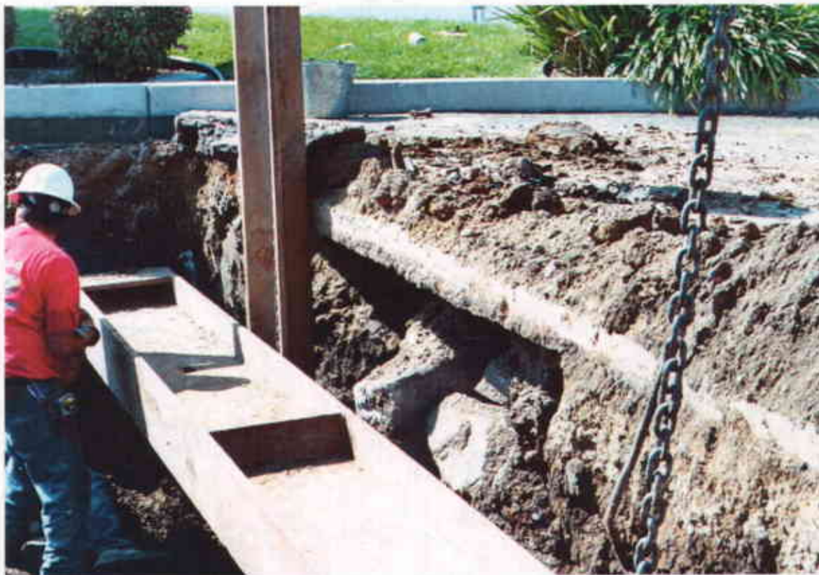
Plate 3: View West showing installation of shoring cross beams into excavation for new UST Area.
