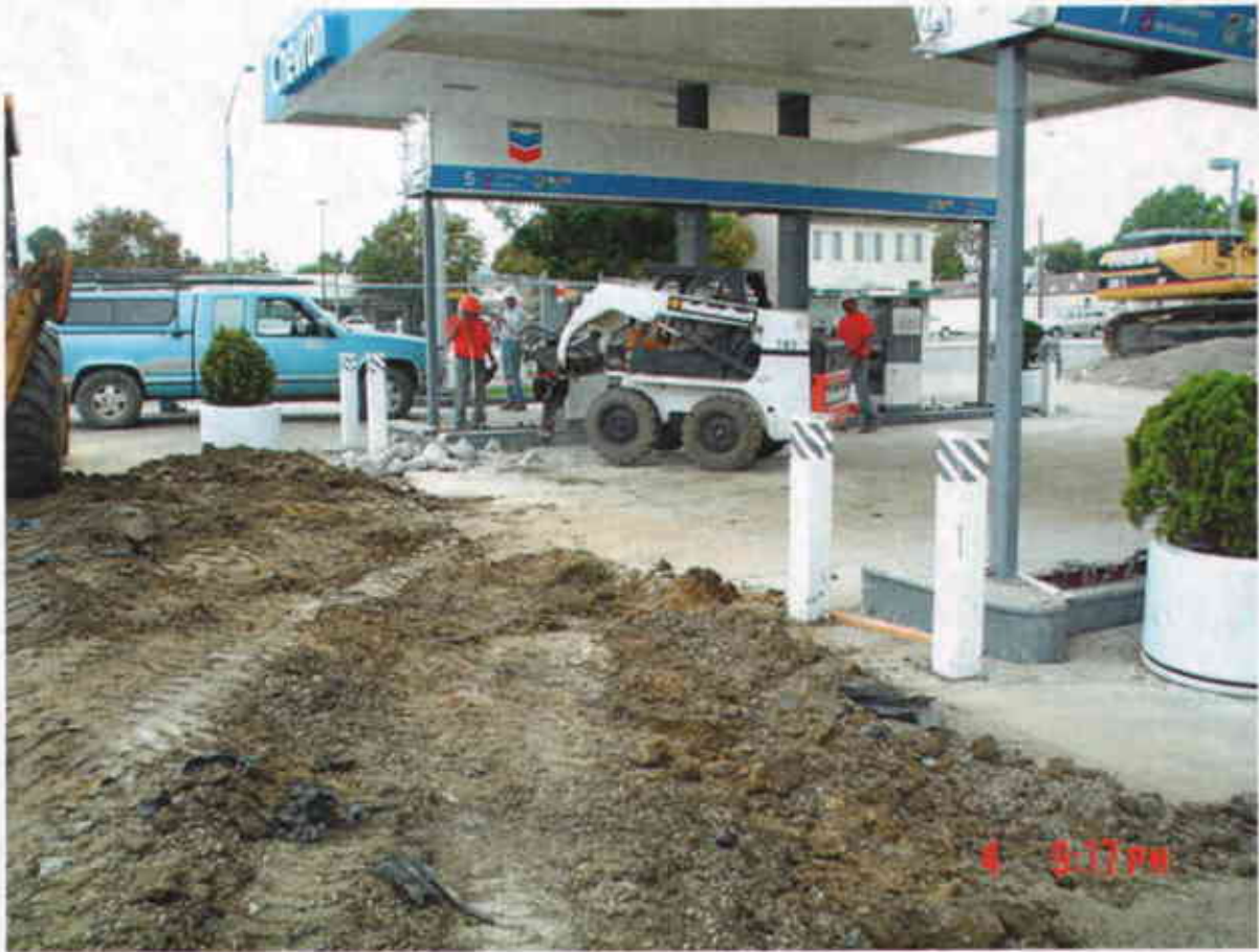
Plate 13: View Northeast showing break-up of concrete slab over product lines.
