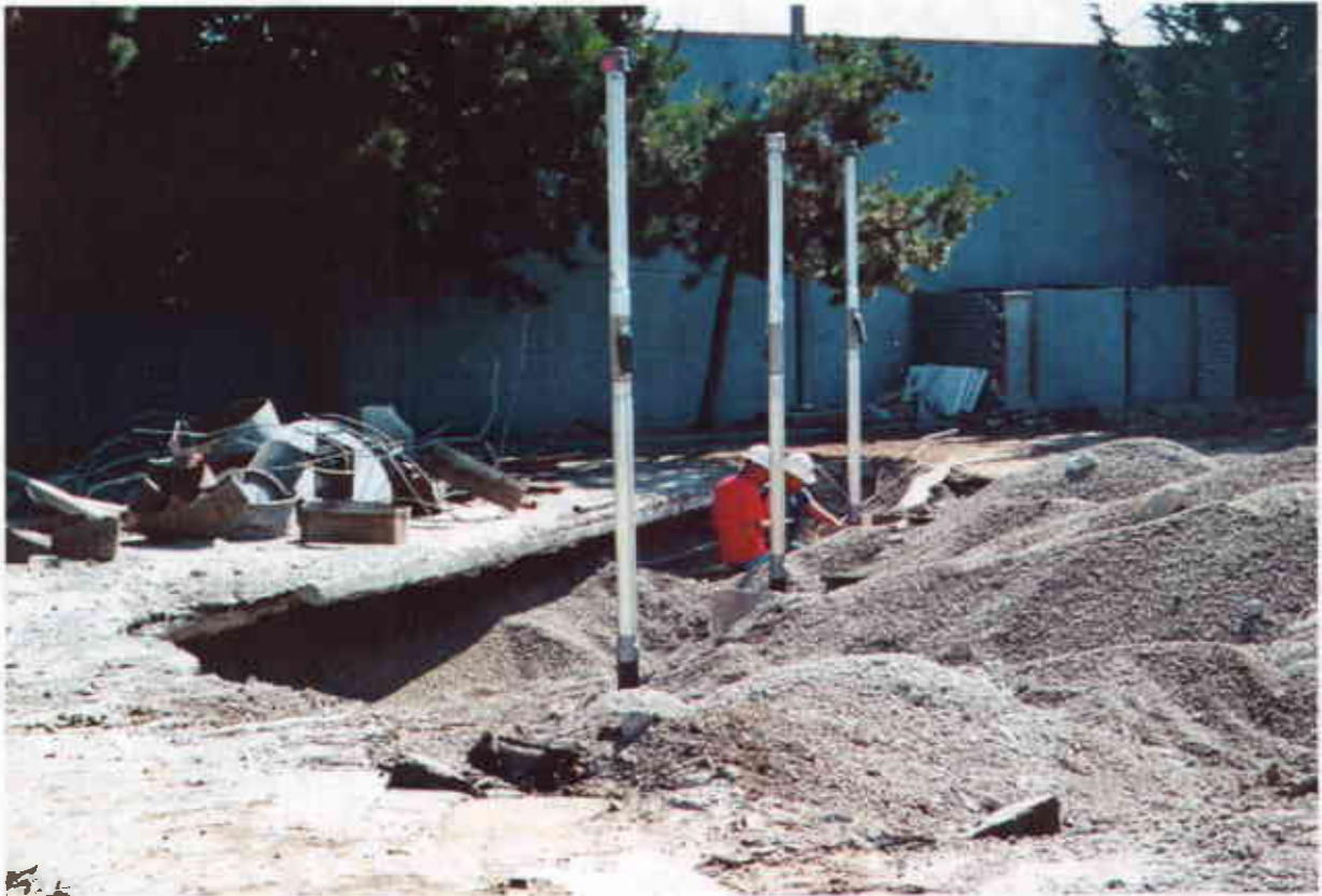
Plate 4: View South showing beginning excavation of existing UST pit and installation of vent pipes.
