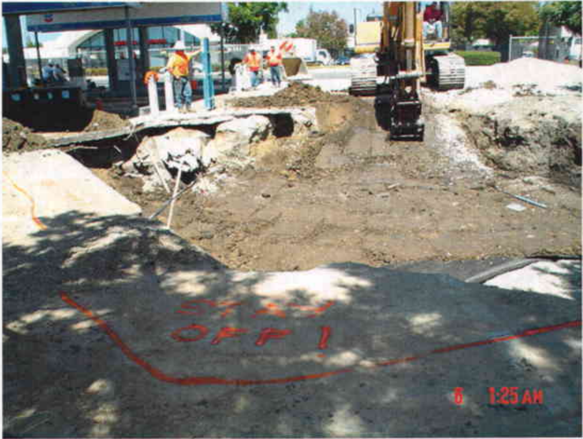
Plate 25: View Northwest showing emplacement and compaction of native-soil fill over filter-fabric covered drain rock.
