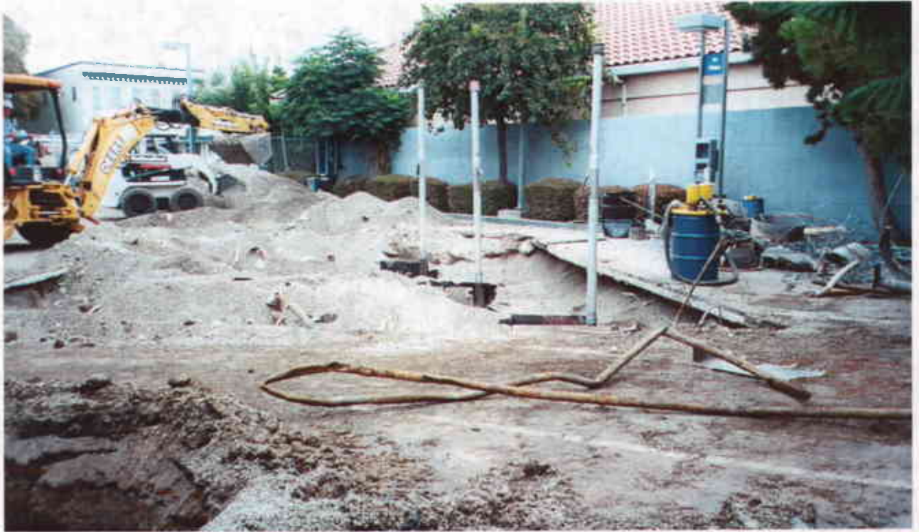
Plate 6: View North showing continued excavation of existing UST pit and metal pipeline excavated from new UST area – shown in foreground.
