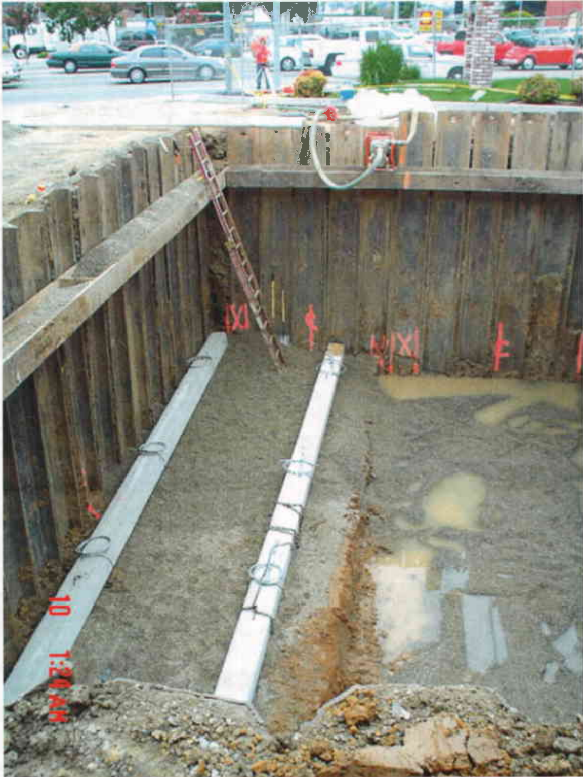
Plate 33: View West showing emplacement of UST foundation beams over pea gravel bedding.
