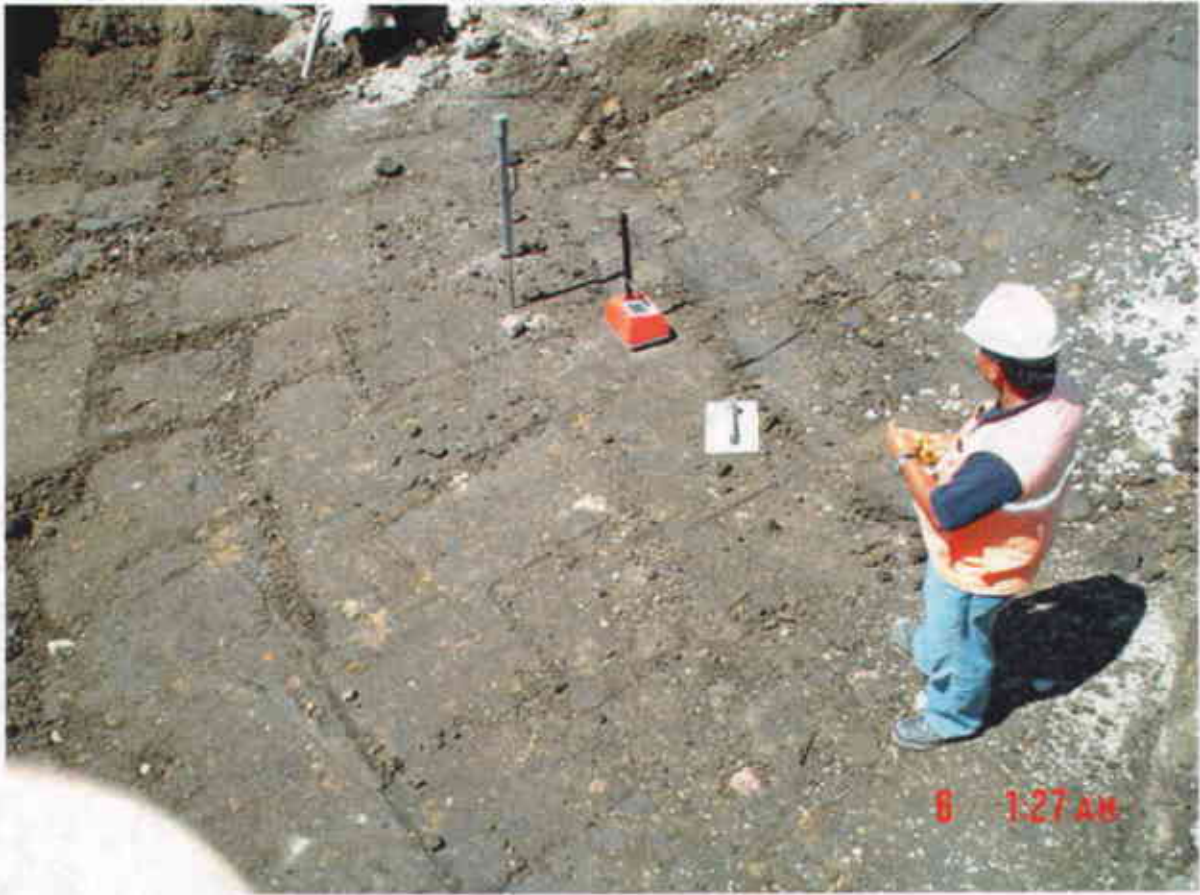
Plate 26: View West down into former UST pit showing compaction testing by BSK Associates.
