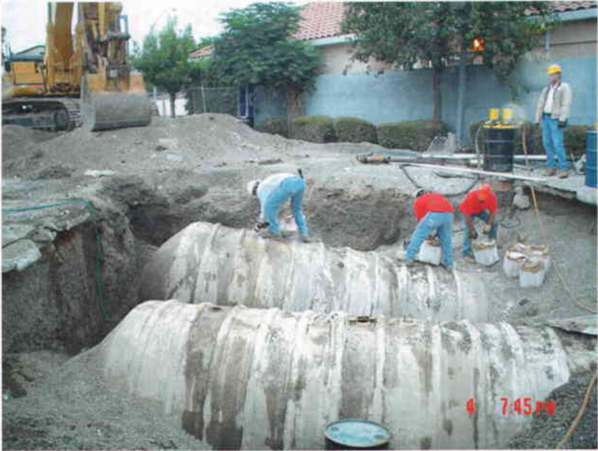
Plate 12: View Northeast showing placement of dry ice into USTs to remove volatile vapors.
