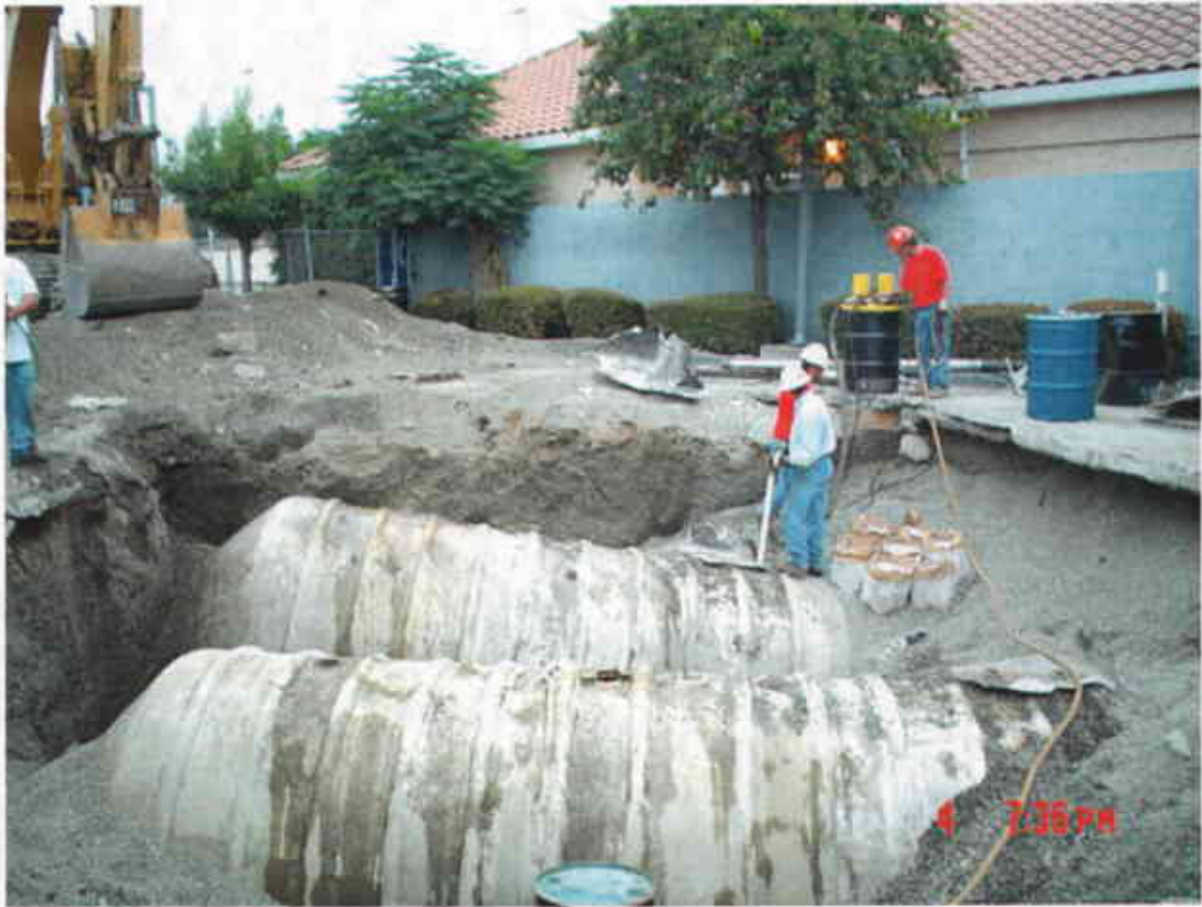
Plate 11: View East showing pumping of remaining fuel from UST #1 with dry ice placed in preparation for purging the USTs of volatile vapors.
