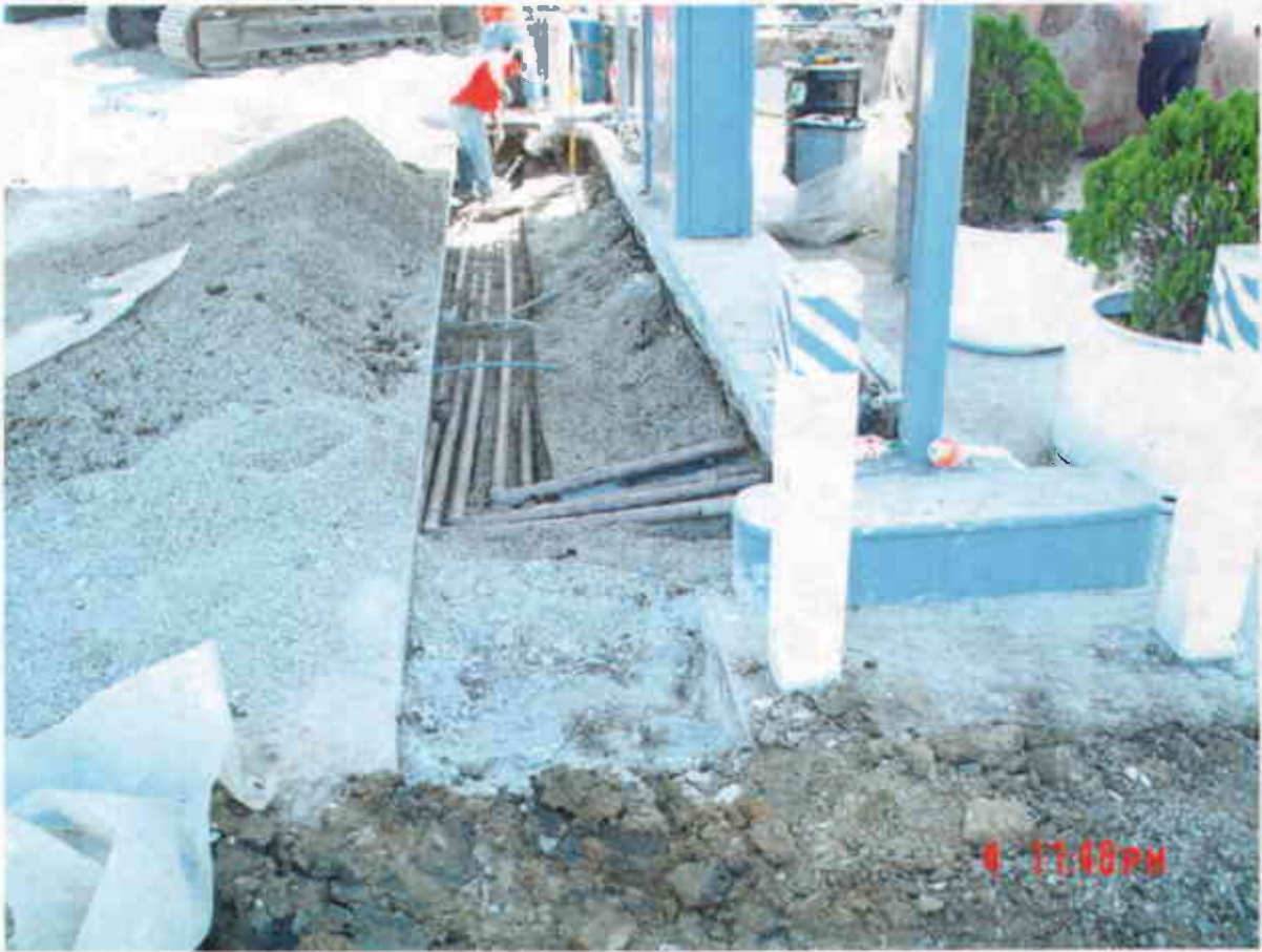
Plate 17: View East showing product lines exposed along north side of south pump island.
