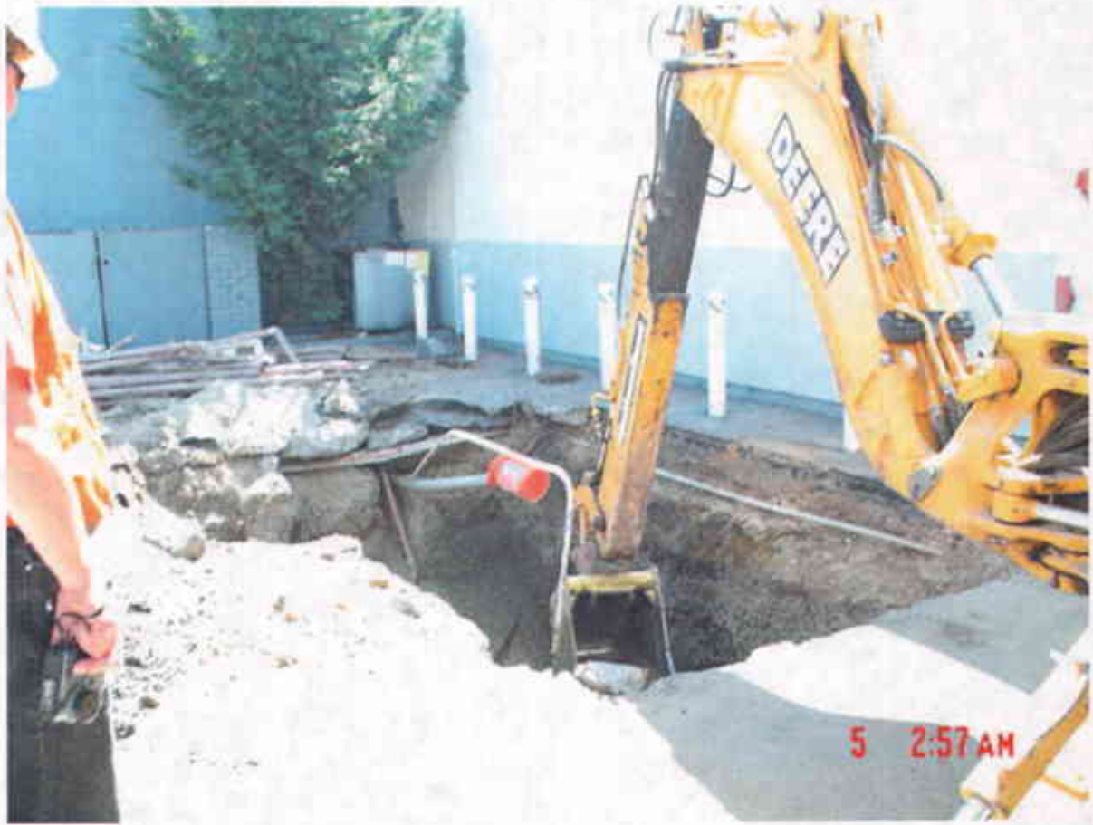
Plate 18: View Southwest showing excavation of waste oil tank pit under oversight of ACHCSA.
