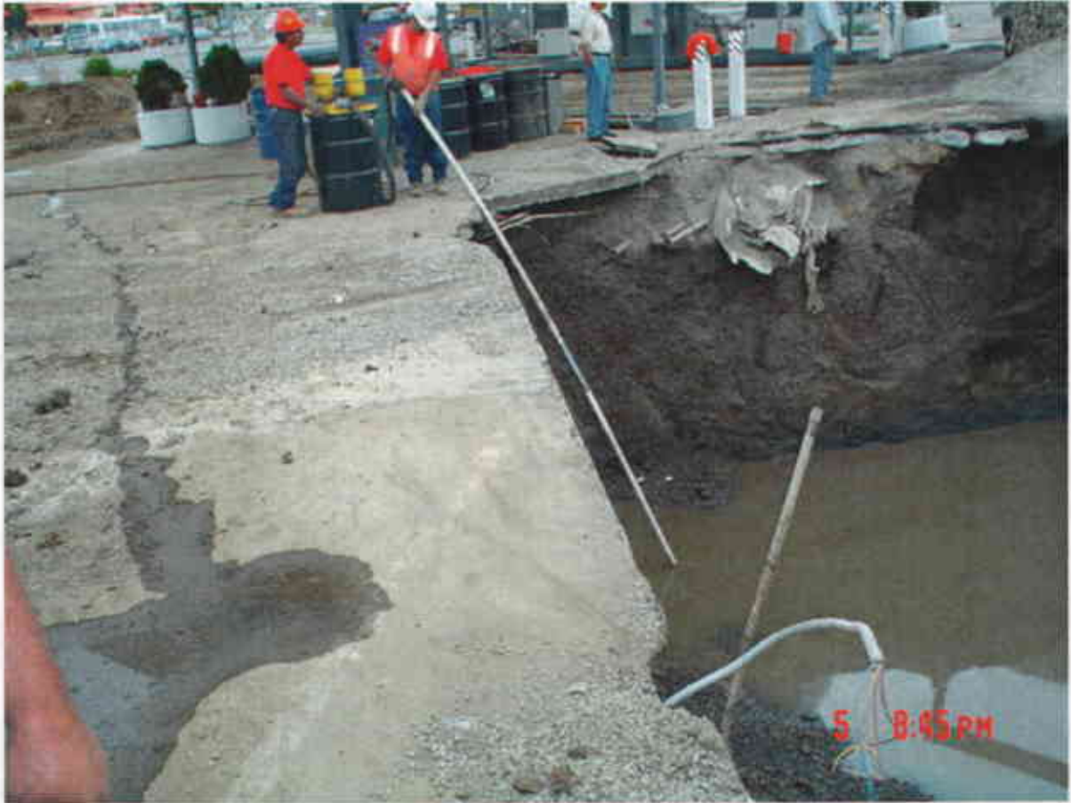
Plate 21: View Northwest showing siphoning of free product from surface of groundwater in former UST pit.
