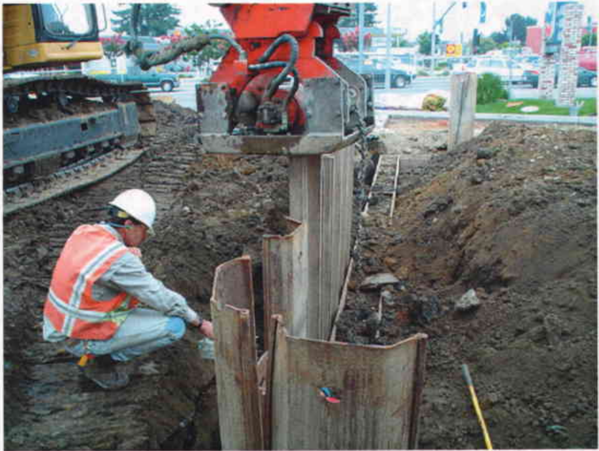
Plate 7: View to West showing driving of shoring around new UST area with SSO checking ambient air with PID.
