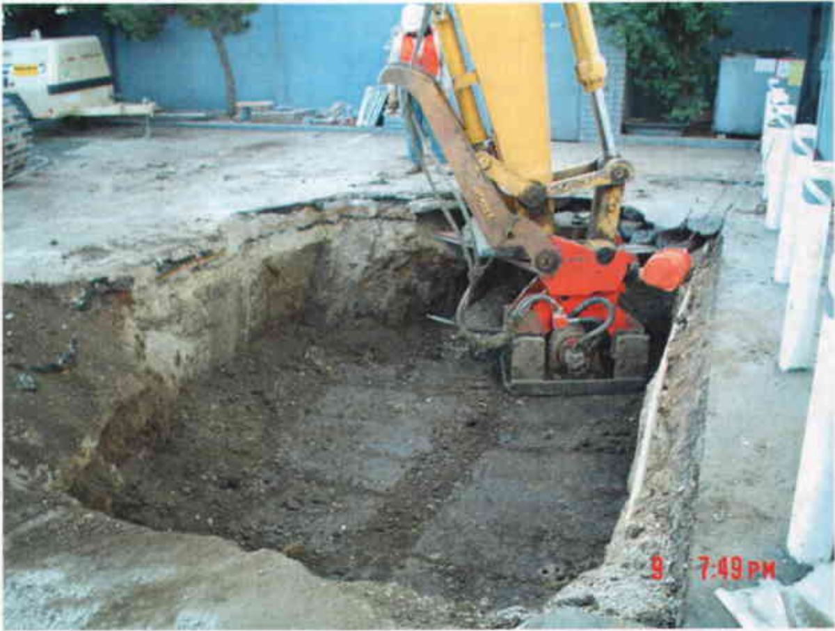
Plate31: View South showing compaction of native soil into former waste oil UST.
