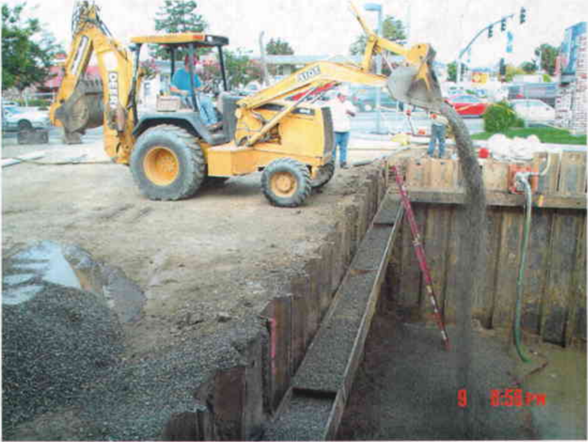
Plate 32: View West showing dewatering of new UST pit during emplacement of bedding gravel for new USTs.
