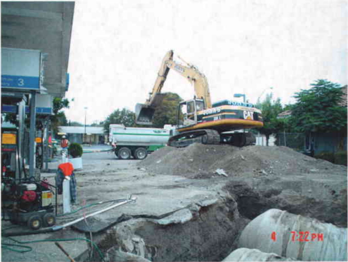
Plate 10: View North showing uploading of excavated pea gravel for off-haul and landfill disposal.
