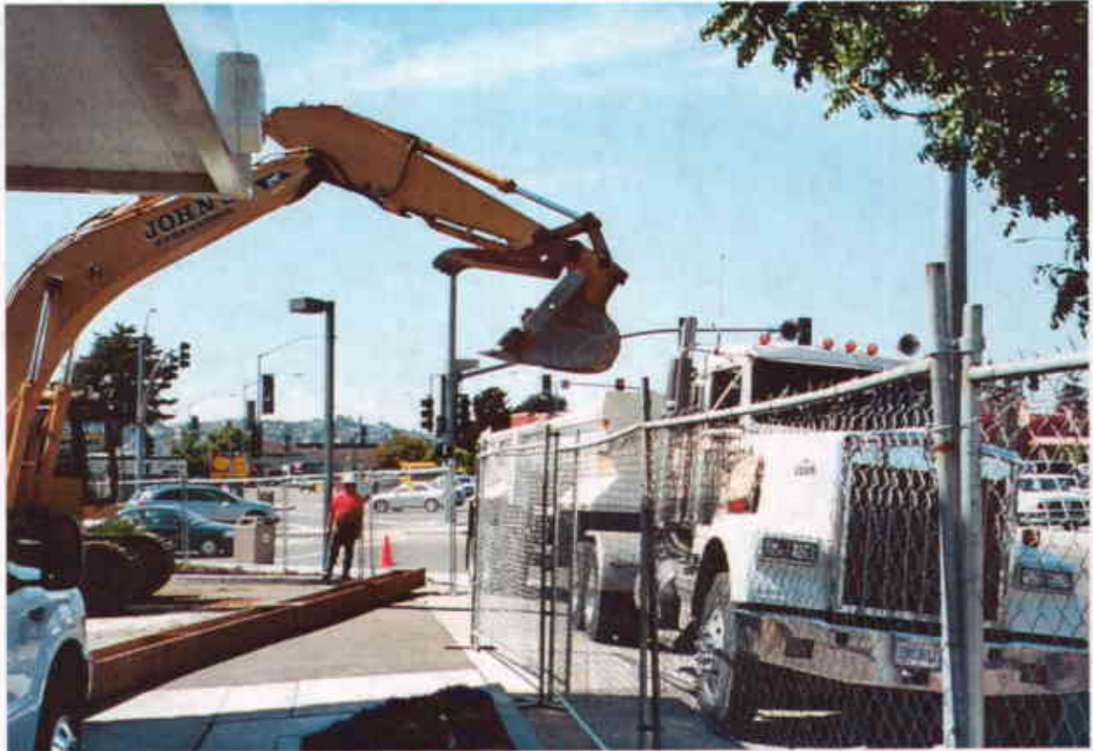
Plate 1: View West showing excavation and uploading of native soil from new UST area.
