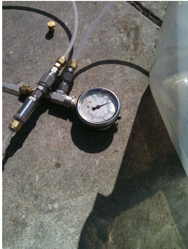
Plate 30. Shut-in test showing continuous vacuum held for two minutes
