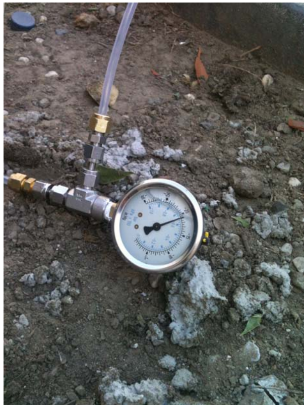
Plate 26. Shut-in test showing continuous vacuum held for two minutes
