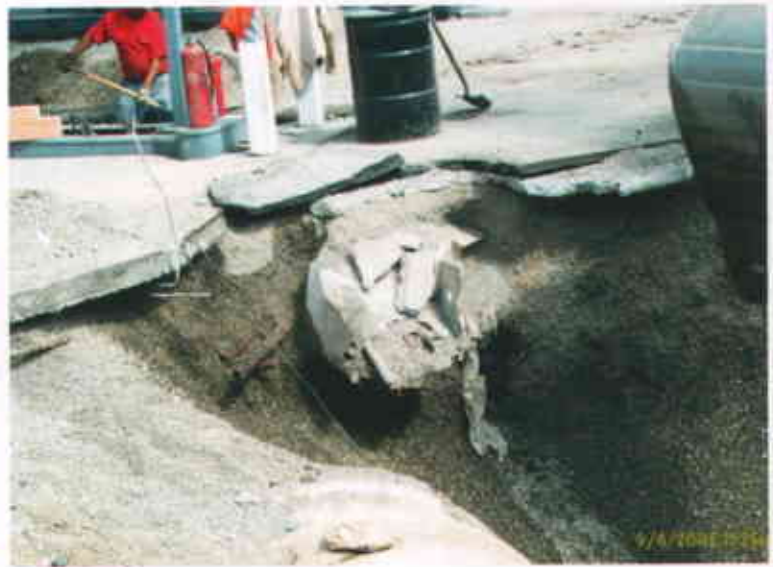
Castro Valley Chevron 3519 Castro Valley Boulevard Castro Valley CA 94546 September 4, 2003 SW FRP Piping junction back to tank field
