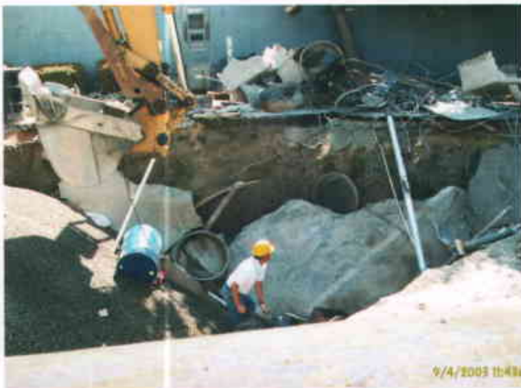
Castro Valley Chevron 3519 Castro Valley Boulevard Castro Valley CA 94546 September 4, 2003 Cave-in of soil, asphaltic cement and tank equipment
