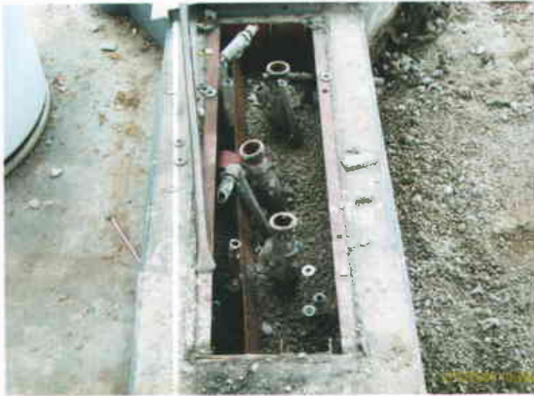
Castro Valley Chevron 3519 Castro Valley Boulevard Castro Valley CA 94546 September 4, 2003 Former under dispenser piping connections
