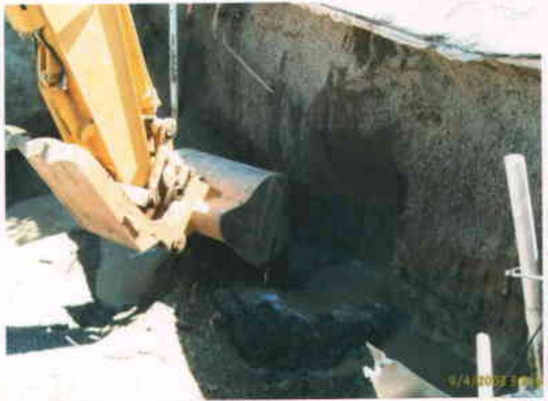
Castro Valley Chevron 3519 Castro Valley Boulevard Castro Valley CA 94546 September 4, 2003 Soil water interface sampling in former tank pit
