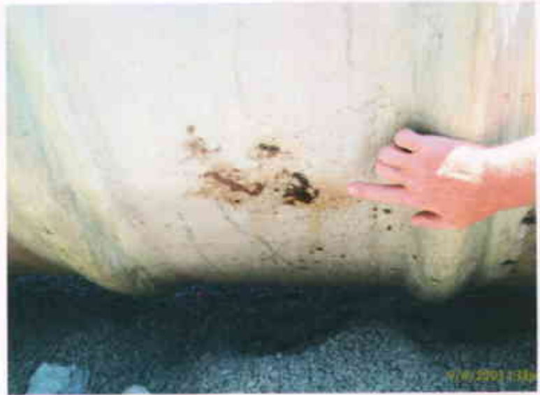
Castro Valley Chevron 3519 Castro Valley Boulevard Castro Valley CA 94546 September 4, 2003 Insignificant stain, not a leak in tank
