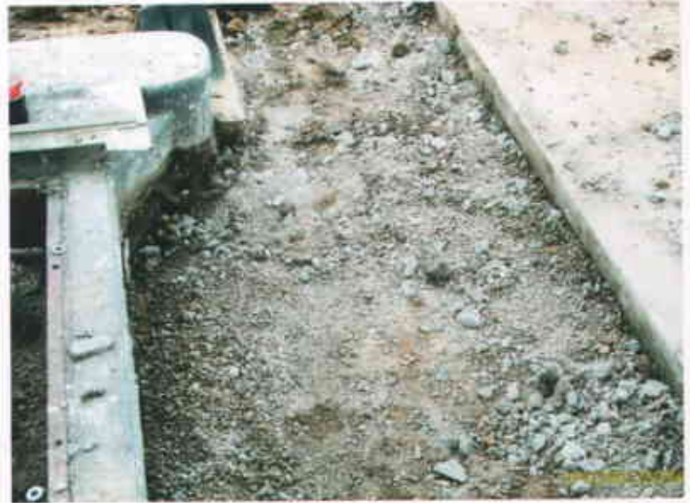
Castro Valley Chevron 3519 Castro Valley Boulevard Castro Valley CA 94546 September 4, 2003 concrete saw cut for removal of piping
