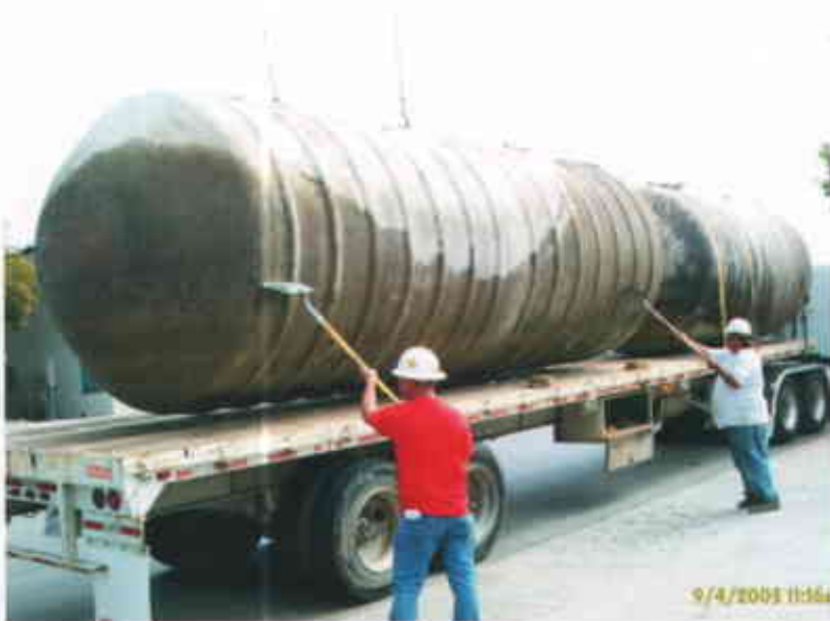
Castro Valley Chevron 3519 Castro Valley Boulevard Castro Valley CA 94546 September 4, 2003 SW FRP Fuel Tanks loaded for disposal at ECI
