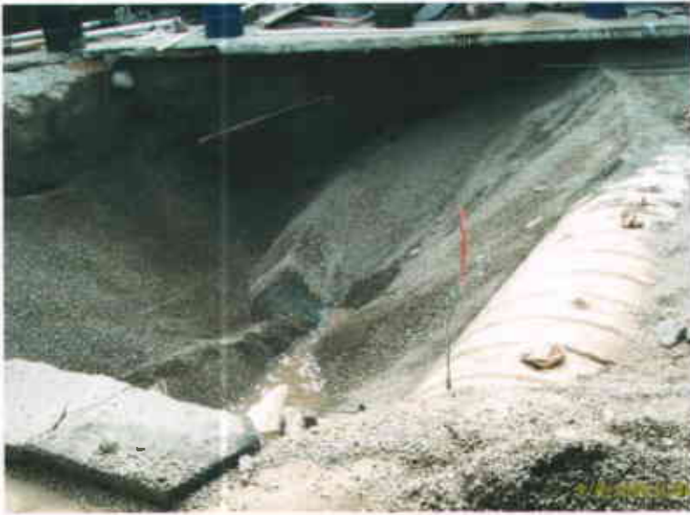
Castro Valley Chevron 3519 Castro Valley Boulevard Castro Valley CA 94546 September 4, 2003 Tank excavation for "old tanks"
